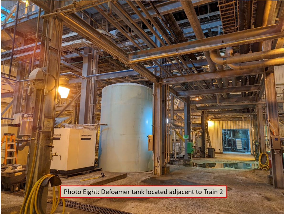
Photo Seven: Leaking heat exchangers for Train 2, bicarb reports to in floor sump
