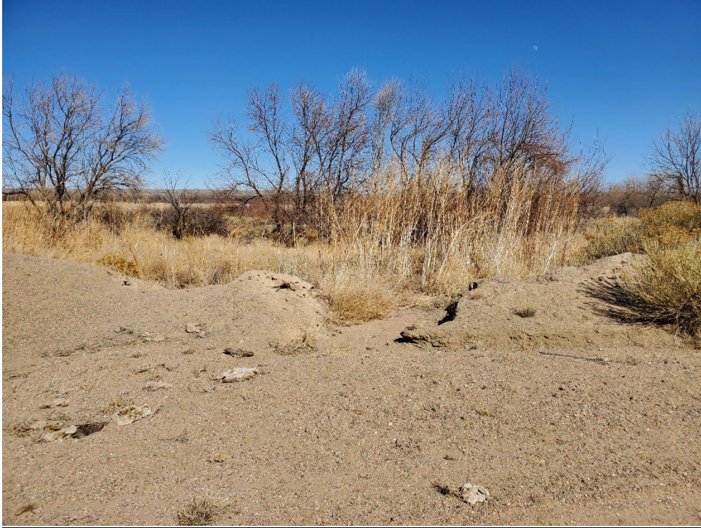
Photo 3: Looking north at northern border of western Phase 1 at eroded berm
