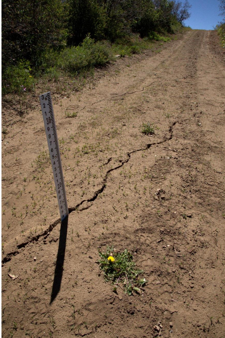
Figure 2: East-Southeast view of subsidence crack diagonal across road on Traverse C-C' located over the E14 Headgate, between Crosscuts 22 and 21.
