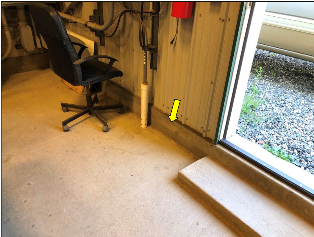
Photo 22. Closer view of floor of water treatment plant, showing 8 inch high concrete berm (indicated) installed around edge of floor. This berm serves as secondary containment for the plant, to contain at least 110% of the maximum storage capacity of all primary containers inside the building holding hazardous chemicals.
