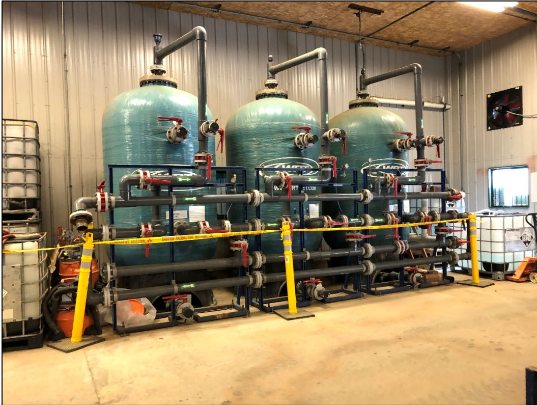
Photo 17. Closer view of IX treatment system inside water treatment plant (along northern wall), consisting of 3 tanks. According to operator, only one tank is typically used at this time, mainly for polishing after primary treatment through RO system.
