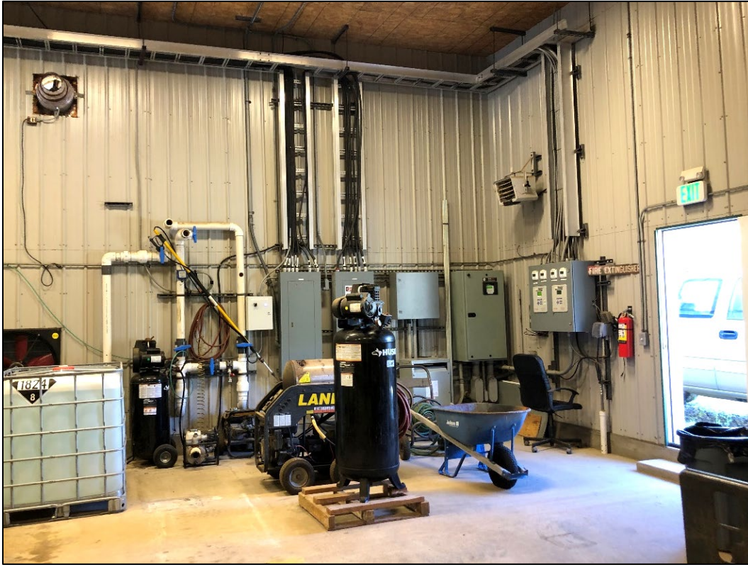
Photo 21. View of main electrical panel located in western corner of water treatment plant.
