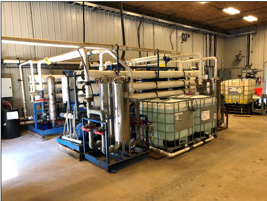
Photo 18. Closer view of RO treatment system inside water treatment plant (along southern wall). This is the primary treatment system for water pumped from the mine workings.
