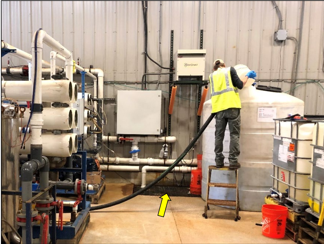
Photo 19. View of mine pump (at center), anti-scale tank (at right), and sump drainage area (indicated) inside water treatment plant (along southern wall). Any fluids captured by sump system are directed to mine workings.
