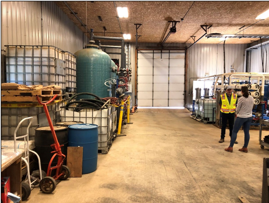
Photo 16. View looking southeast inside water treatment plant, showing IX system and resin storage area (at left) and RO system (at right). Note approx. 12 foot x 17 foot garage door at end of building, with concrete floor ramp.
