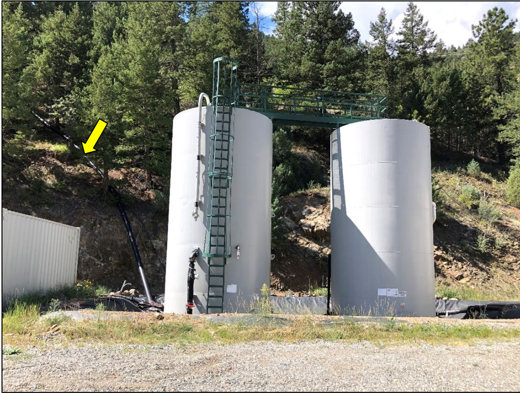
Photo 15. View looking west at reactor tank and backfill slurry tank which sit inside a lined secondary containment basin. Note pipeline (indicated) which runs from dewatering pump inside Jeffrey Air Shaft (located uphill from plant) for approx. 250 feet down to tanks.
