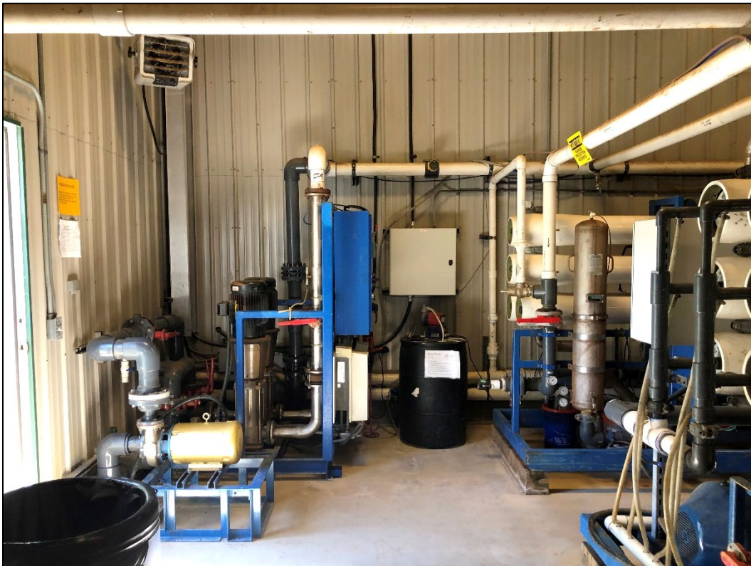
Photo 20. View of backfill pump, booster pumps, backfill pump VFD, and barium chloride drum (at center) located in southern corner of water treatment plant. Note portion of RO system visible at right.
