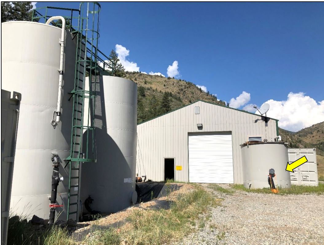
Photo 14. View looking northwest at southeastern side of water treatment plant (on top of mesa). Note reactor tank and backfill slurry tank (in foreground) which sit inside a lined secondary containment basin, and clean water tank (indicated in background).
