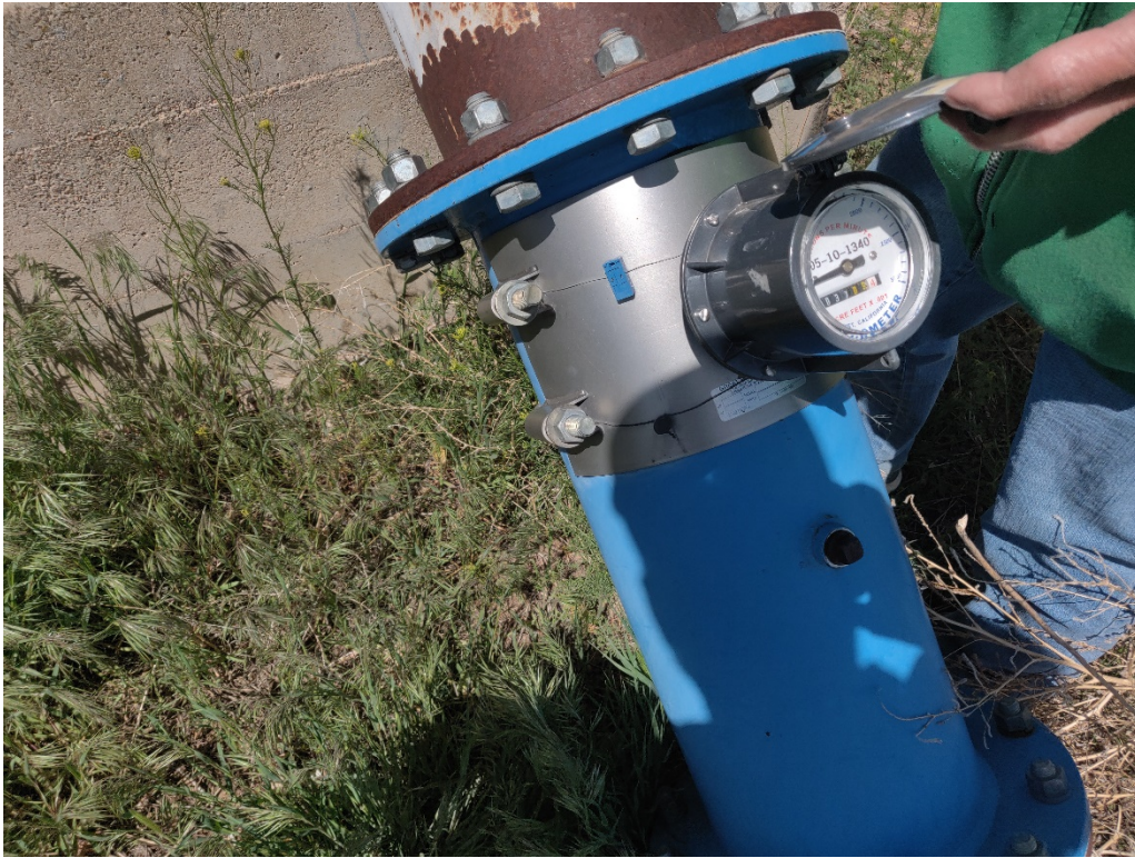
View of the flow meter installed on the well outlet pipe
