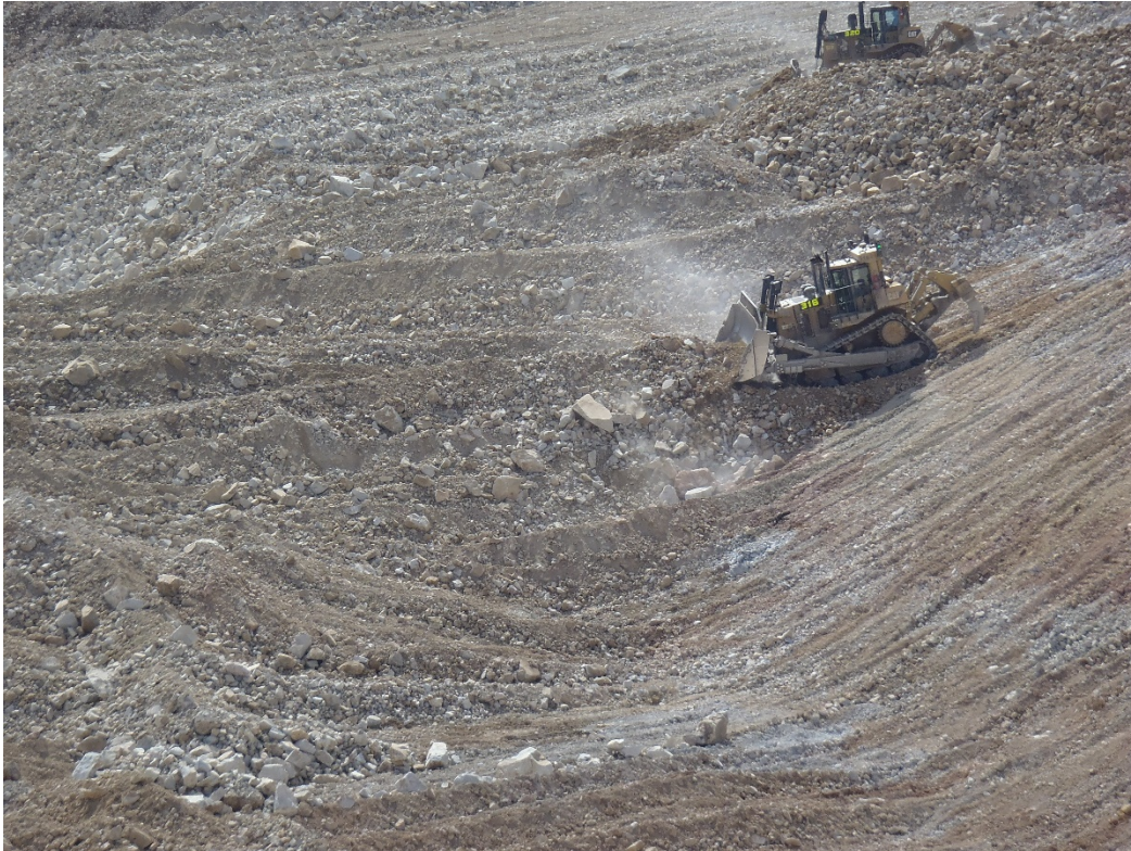
Photo 4. Oversize rock in Turkey Ridge material – to be wasted on ECOSA
