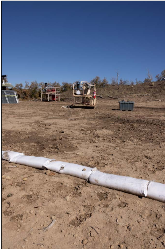
Figure 7. Northward view during the fall 2021 field visit of the same approximate area shown in Figure 6. Note that the previously-observed subsidence cracks are no longer visible.
