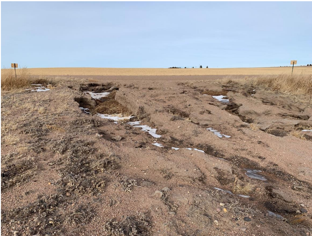
Photo 7 – Gullies in area 1
