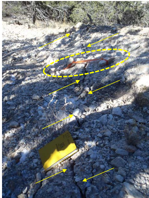
Photo 5. Tension crack viewed in access road/dozer trail, ~150 east of dozer (looking west). {Note: orange tape (circled) anchored on each end by rocks straddles tension crack}
