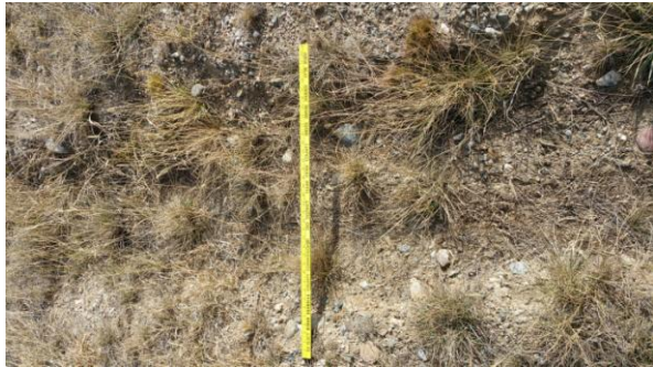
Photo 12. Asphalt surface with sparse growth.
