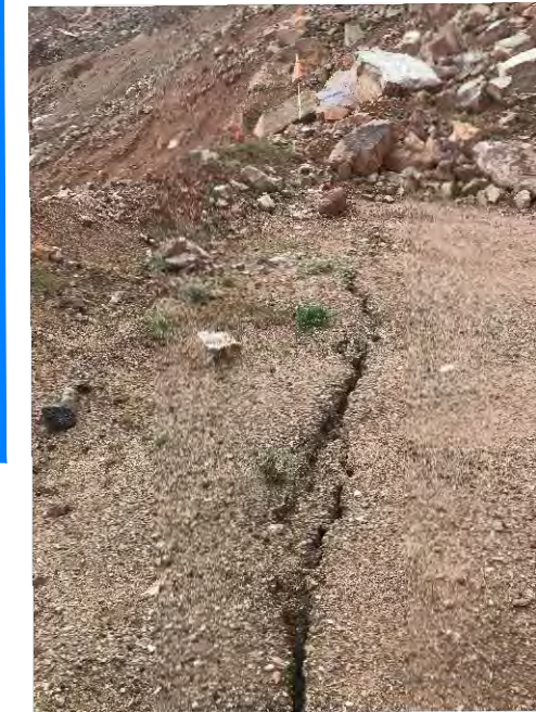
2. CRACKING NEAR PRODUCTION FLOOR
