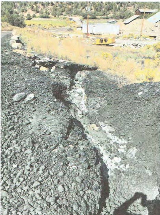
Pic. 2 – Erosion between haul road/NW corner of lower waste pile.
