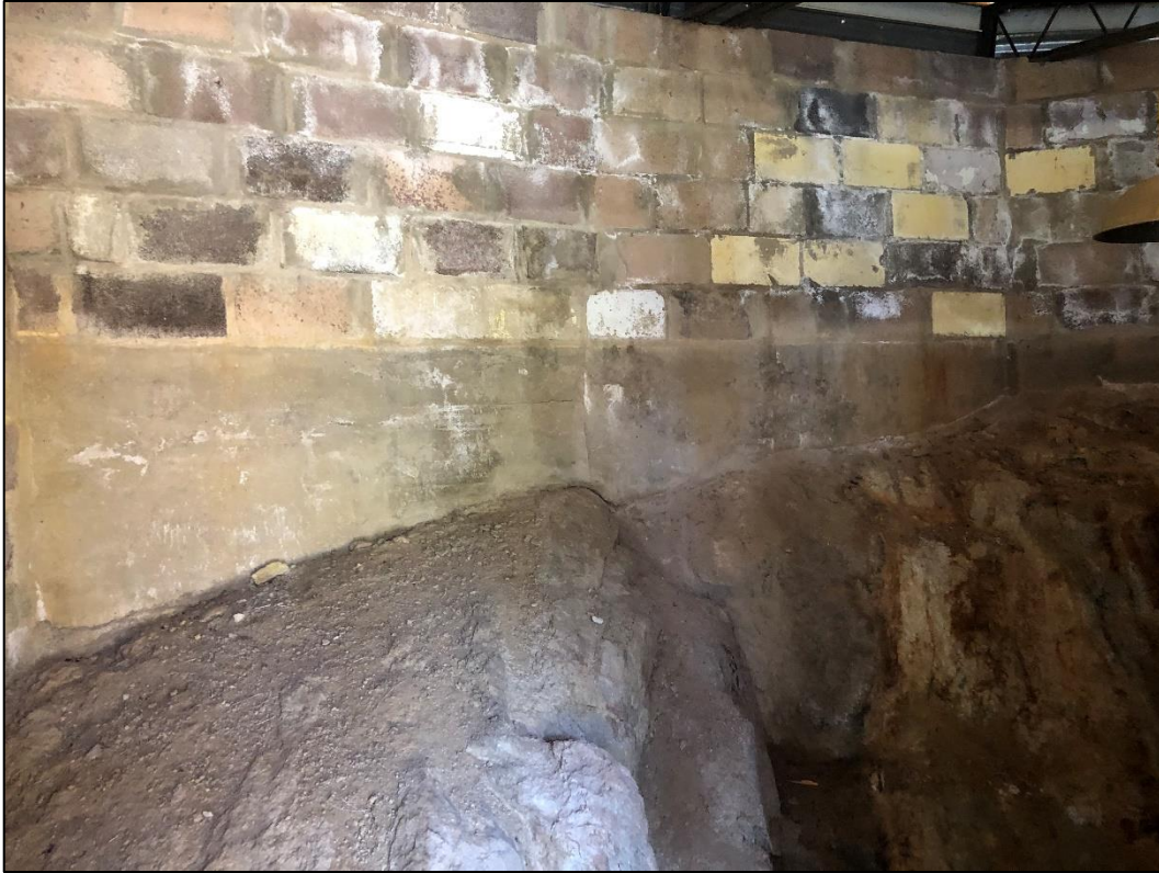
Photo 11. View inside winch house, showing concrete wall built into bedrock which would need to be demolished and removed from site unless reclamation plan is revised to leave winch house. Hole inside building (at bottom right) must be capped or backfilled for reclamation.
