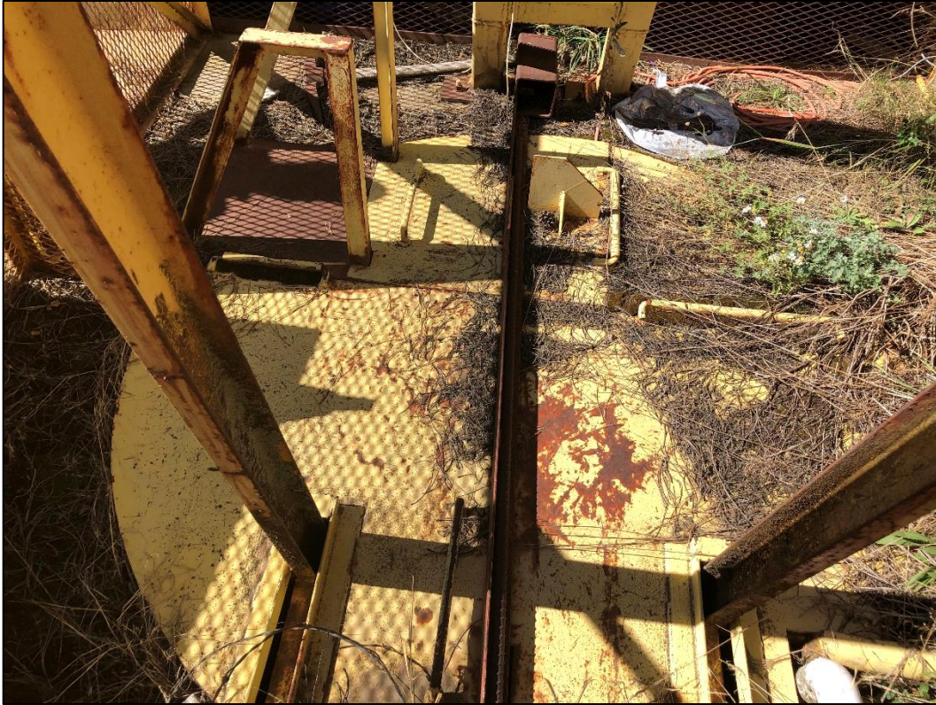
Photo 9. View of Phil Sheridan Shaft collared in concrete slab, and capped and secured by covered locking device. Shaft area is enclosed by metal fencing.
