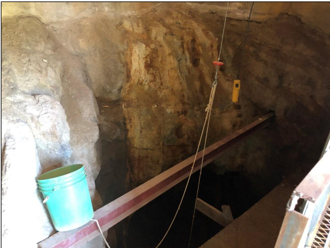
Photo 10. View inside winch house, showing hole in bedrock which must be capped or backfilled for reclamation.
