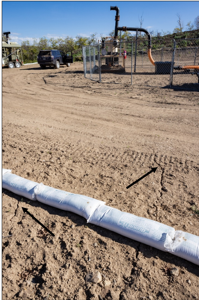
Figure 6. Northward view during the spring 2021 field visit of a two smaller subsidence cracks on the southern portion of the MVB SS1-6 pad (see black arrows).
