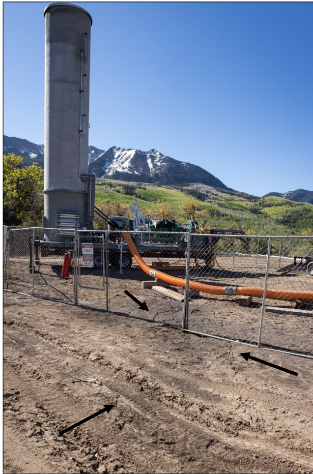
Figure 5. Southeastward view during the spring 2021 field visit of two additional sub-parallel sets of cracks located within and north of the fenced area around the wellhead on the MVB SS1-6 pad.
