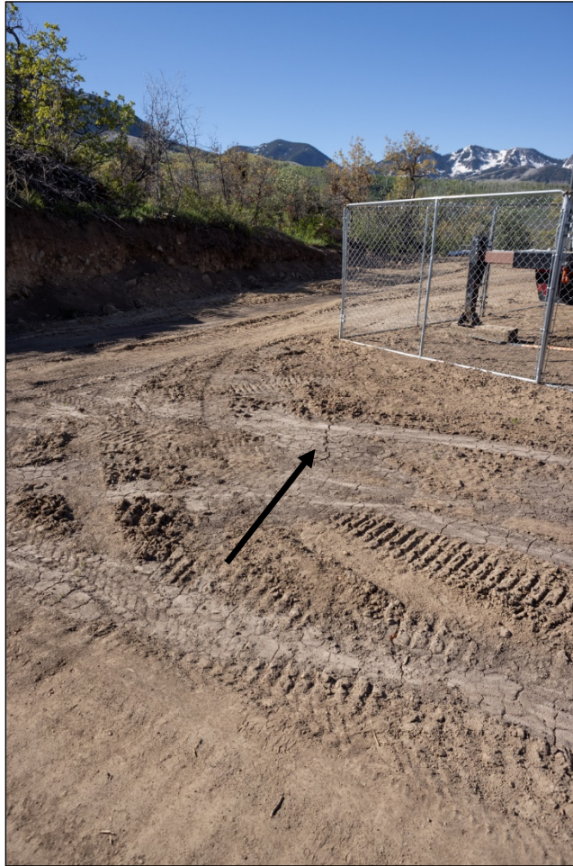
Figure 4. Southward view during the spring 2021 field visit of one the subsidence cracks located in the northeastern portion of the MVB SS1-6 pad. This particular crack is visible directly beneath the corner post of the fence as indicated by the black arrow. Several sub-parallel cracks (about 6-8 feet apart) were observed at this location with an orientation of about N20-40°W.
