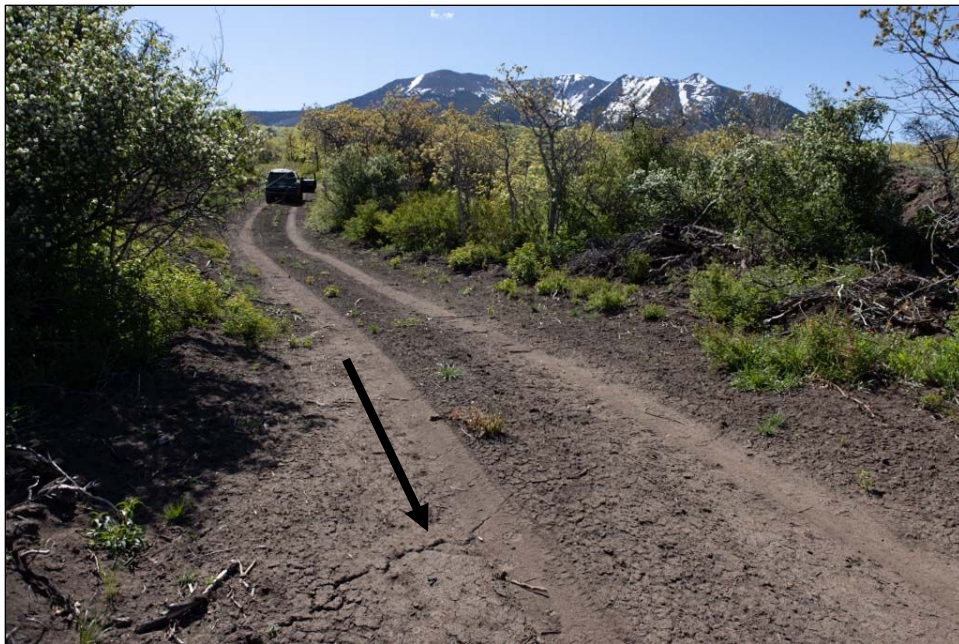
Figure 8. Eastward view during spring 2021 of a second subsidence crack located approximately 30 feet east of the one shown in Figure 7 and with smaller maximum dimensions. Both cracks are most obvious on the north side of the road.
