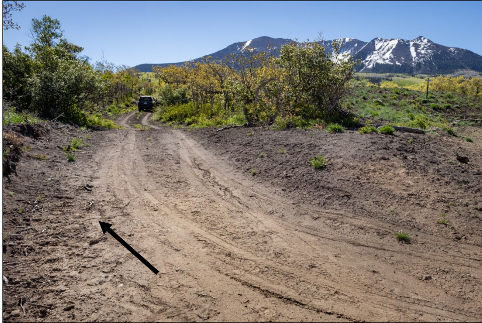
Figure 7. Eastward view during the spring 2021 field visit of a subsidence crack located where the access road meets the MVB SS1-7 pad. This, and nearby cracks on the pad and road are the result of active mining occurring beneath this area.
