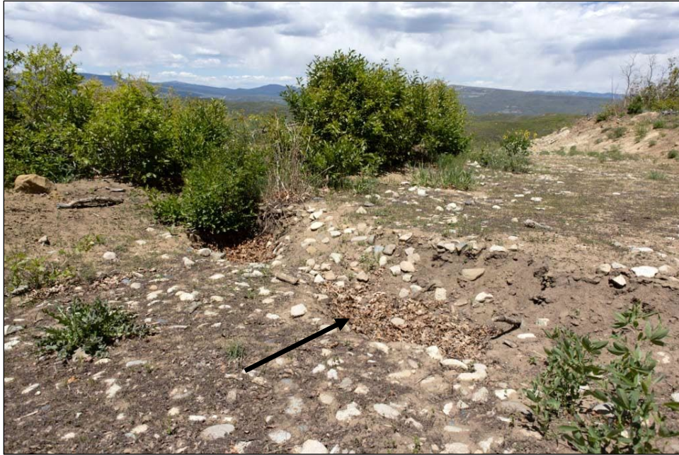
Figure 3. Northwestward view during the spring 2021 field visit of a subsidence crack first observed during our spring 2019 field visit. The 6-inch elevation offset from north to south (right to left) is still present, but materials have filled the deepest portions of the crack and rounded the edges. This location is approximately 1,000 feet north of the MVB E6-14 pad.
