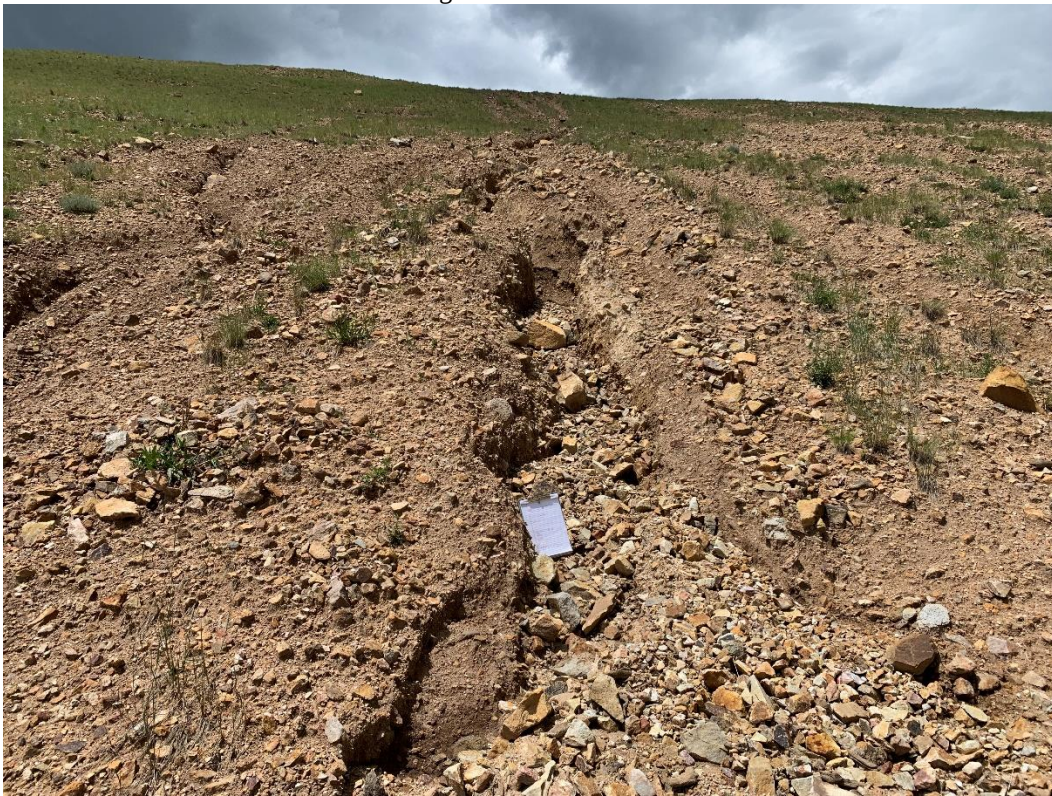
Photo 13 – Erosion and gullies on the east side of the Altman Backfill
