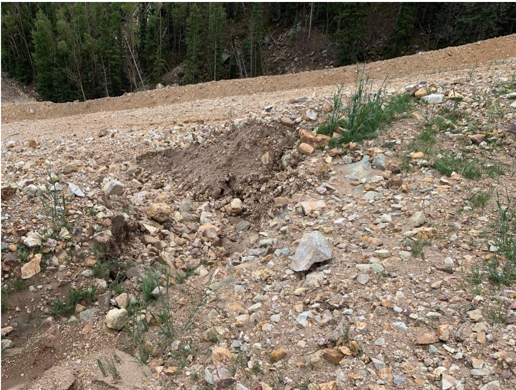
Photo 9 – Gully at the end of the upper contour ditch, perimeter ditch in background
