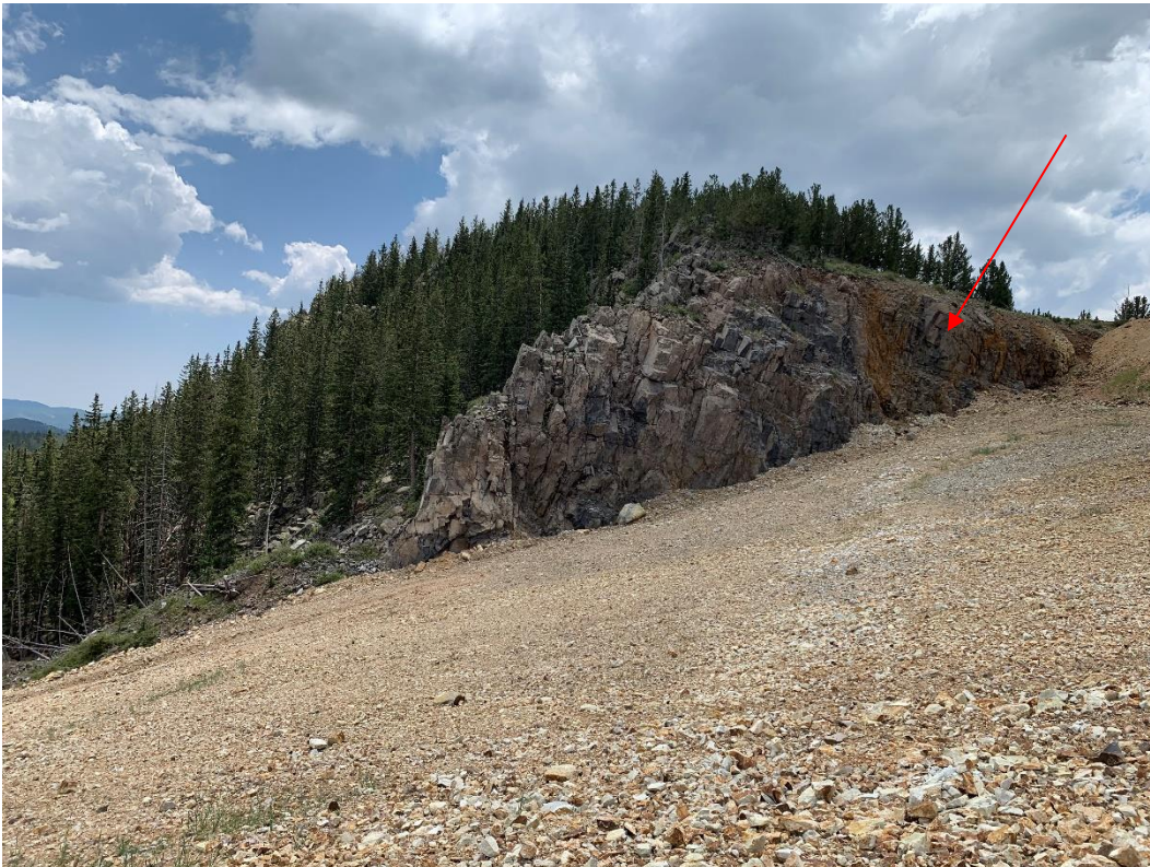
Photo 7 – Highwall area that has not been backfilled and needs a fence.
