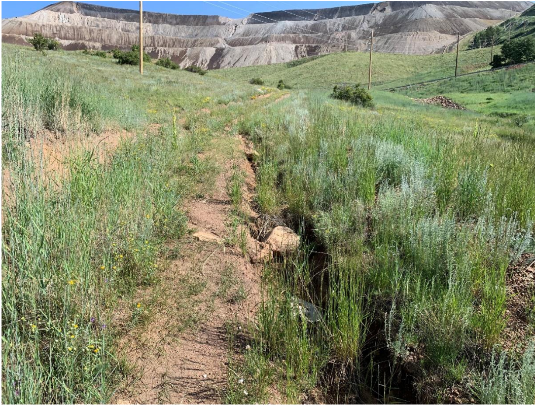
Photo 2 – Gully on GM-19 on northeast access road
