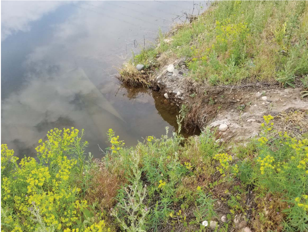
Photograph #2. Erosion gully on north reservoir created by inlet water discharge.
