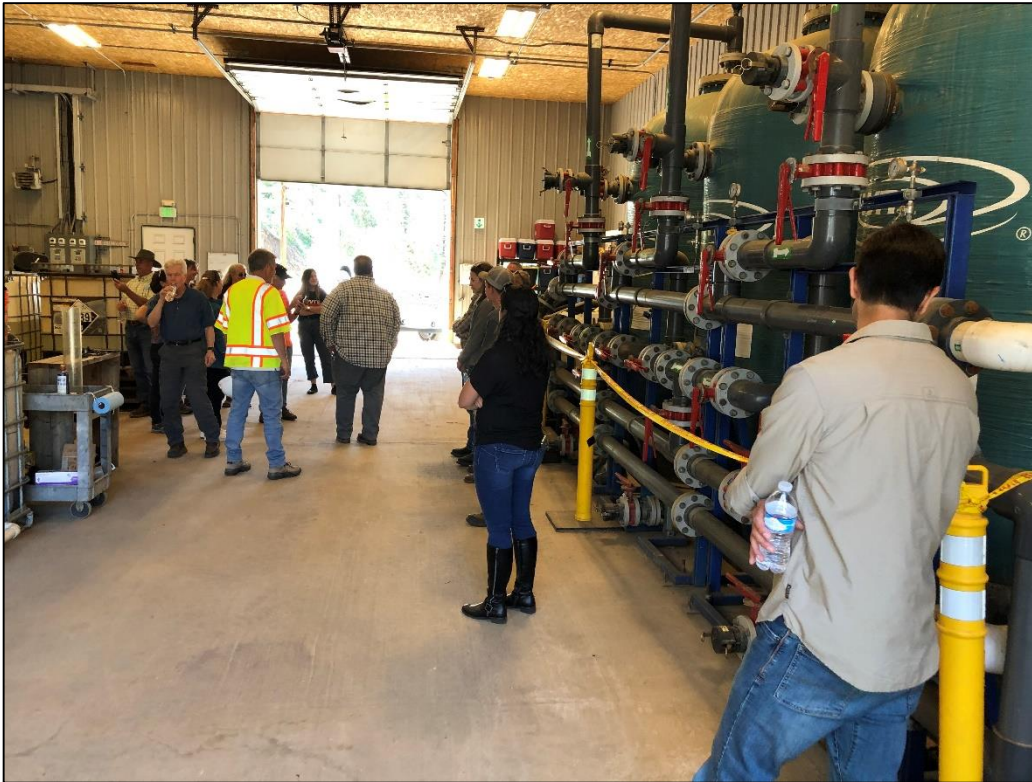
Photo 11. View looking inside water treatment plant located on top of mesa. This plant treats water pumped from the mine pool, any alluvial water collected in the downgradient sump, and any surface water that comes into contact with contaminated valley soils within the mine disturbance area. Treated water is discharged at operator's permitted outfall (SW-BPL) on Ralston Creek.
