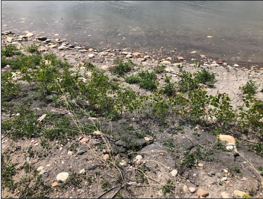
Photo 21. Closer view of southeastern shoreline of North Reservoir, graded mostly 3H:1V or flatter with very sparse vegetative cover consisting primarily of volunteer cottonwood trees. Operator will need to remove trees, repair any erosion rilling, and reseed shoreline as needed.
