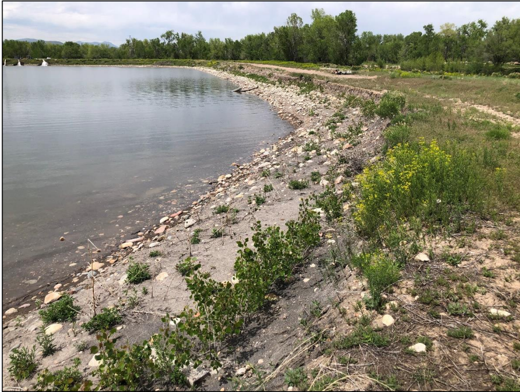
Photo 19. View looking north across eastern shoreline of North Reservoir, graded mostly 3H:1V or flatter with very sparse vegetative cover consisting primarily of volunteer cottonwood trees. Operator will need to remove trees, repair any erosion rilling, and reseed shoreline as needed. Weed control must also be implemented in this area for state-listed noxious weed species.
