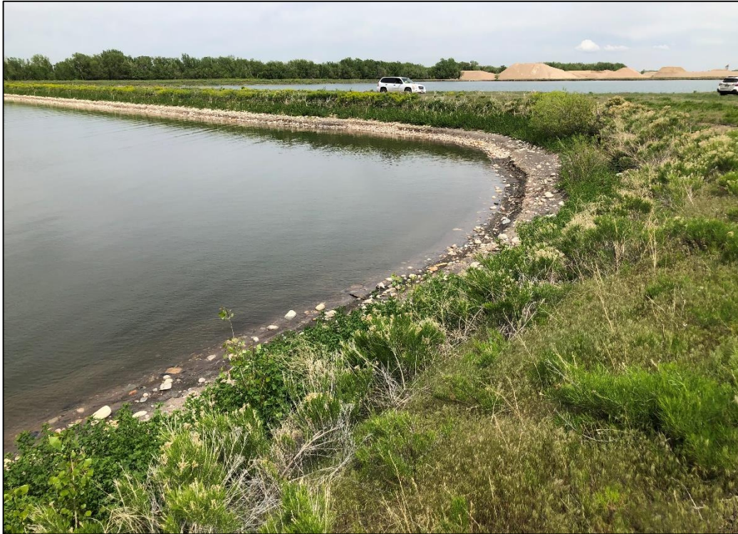
Photo 29. View looking southeast at southern shoreline of North Reservoir, graded mostly 3H:1V or flatter with dense cluster of volunteer cottonwood trees. Operator will need to remove trees, repair any erosion rilling, and reseed shoreline as needed. Weed control must also be implemented in this area for state-listed noxious weed species.
