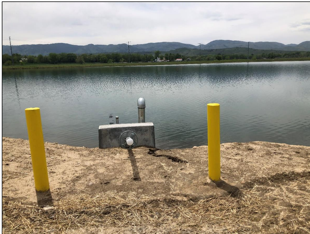
Photo 16. View looking west at outlet structure recently installed at northeastern edge of South Reservoir. The reclamation plan and map need to be updated to address any permanent water management structures installed on the affected lands.
