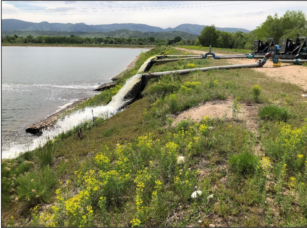
Photo 23. View looking west across northern shoreline of North Reservoir, showing three above-ground pipelines discharging water pumped from river into the reservoir. Note large erosion gullies created along shoreline from this discharge. Operator will need to repair erosion damage and reseed shoreline as needed. Weed control must also be implemented in this area for state-listed noxious weed species.
