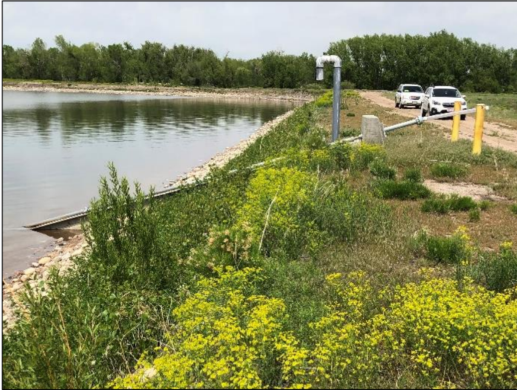
Photo 27. View looking northeast at control structure installed at southeastern edge of North Reservoir. The reclamation plan and map need to be updated to address any permanent water management structures installed on the affected lands. Operator will need to implement weed control plan in this area for state-listed noxious weed species
