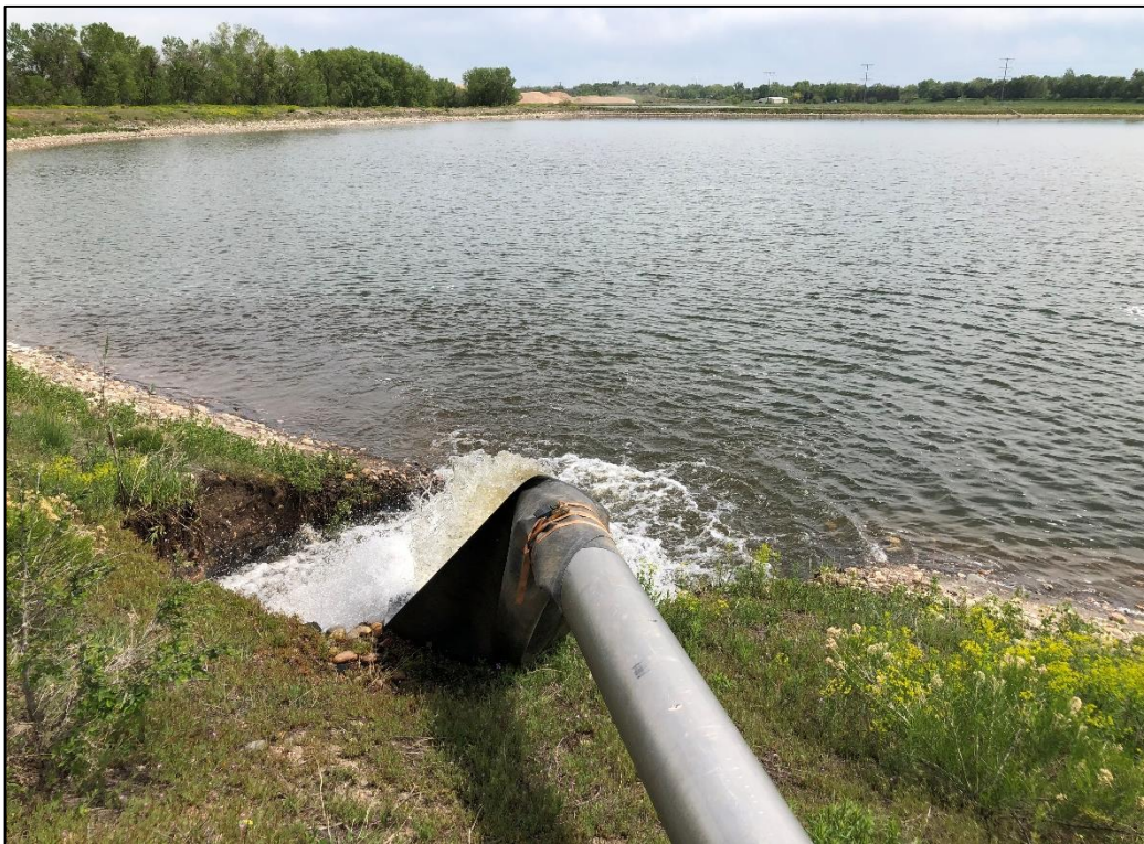
Photo 24. Closer view of pipeline discharging water into North Reservoir along its northern shoreline, showing large erosion gully (approximately 6 feet deep) created along shoreline. Operator will need to repair this erosion damage and reseed shoreline as needed.
