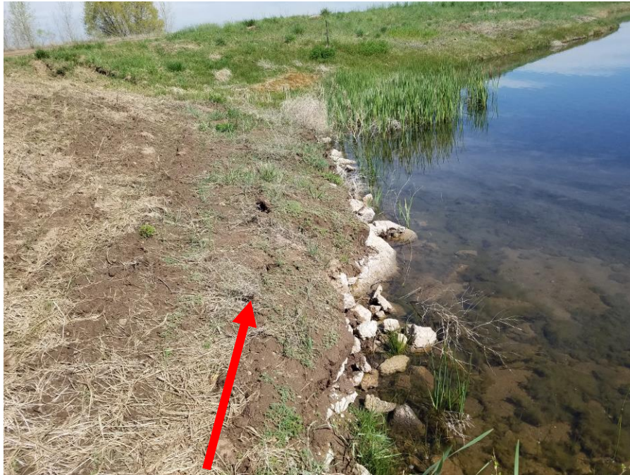
Figure 5. Small crack in the southwest corner of Cell No. 4.
