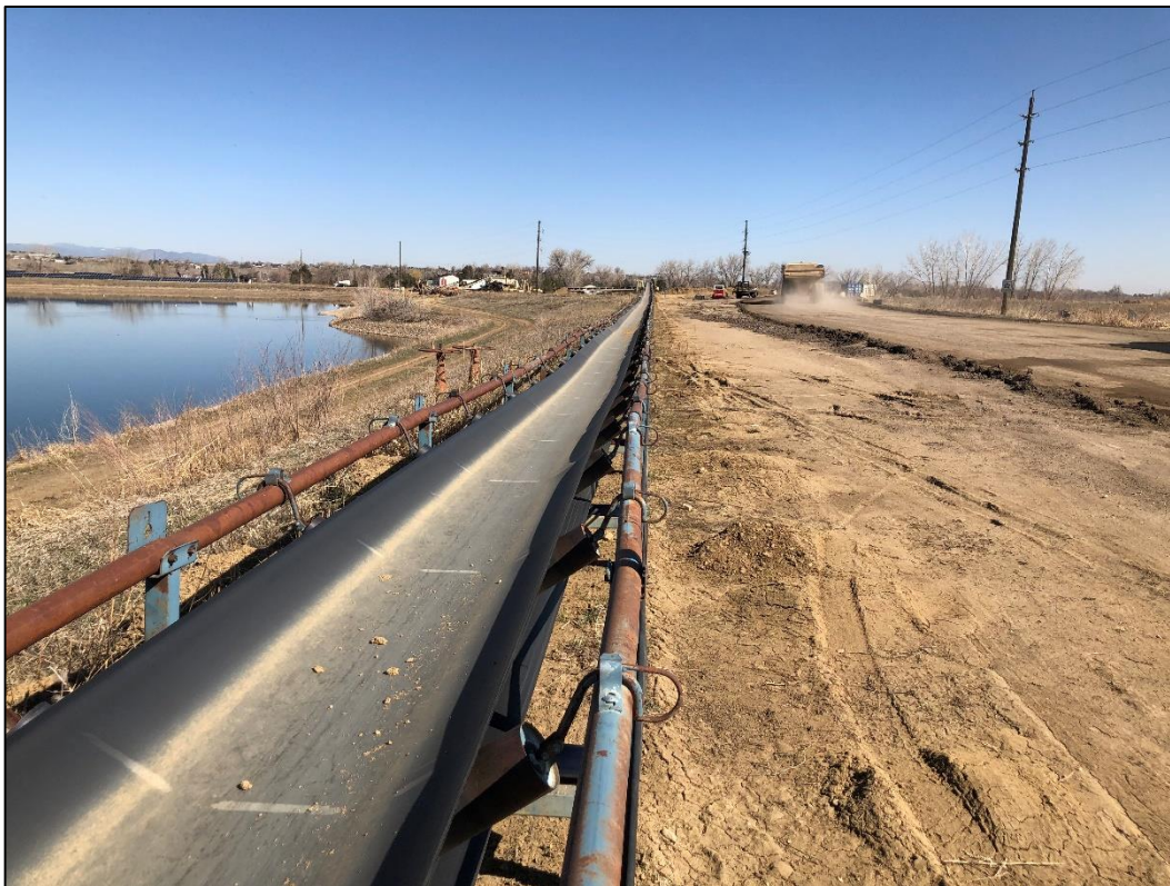
Photo 10. View looking north across conveyor system installed between Reservoir #2 pit (to the south) and processing plant in Reservoir #4 pit (to the north). This system was offline during the inspection, and according to operator, will no longer be used by the operation.
