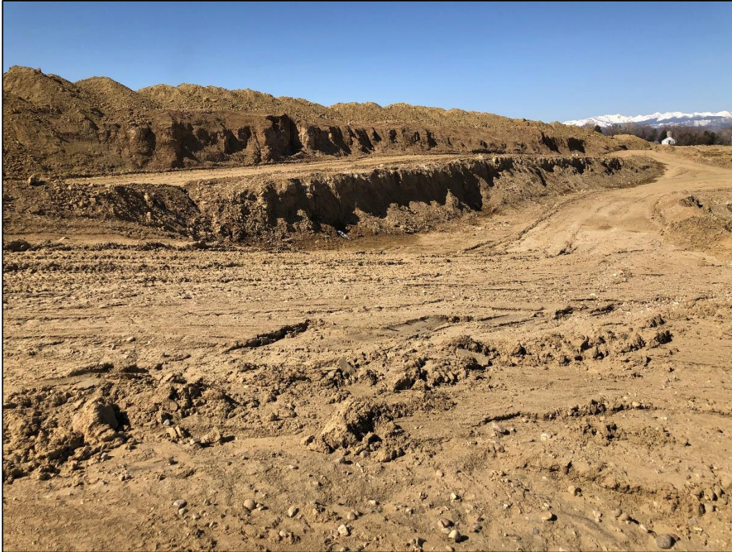
Photo 21. View looking west across southern edge of new (unauthorized) reservoir pit where clay liner has not been installed. Note overburden stockpiles (above pit wall) in storage area south of reservoir.
