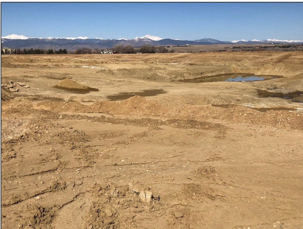
Photo 20. View looking west across new (unauthorized) reservoir pit. Note standing water on pit floor (at right).
