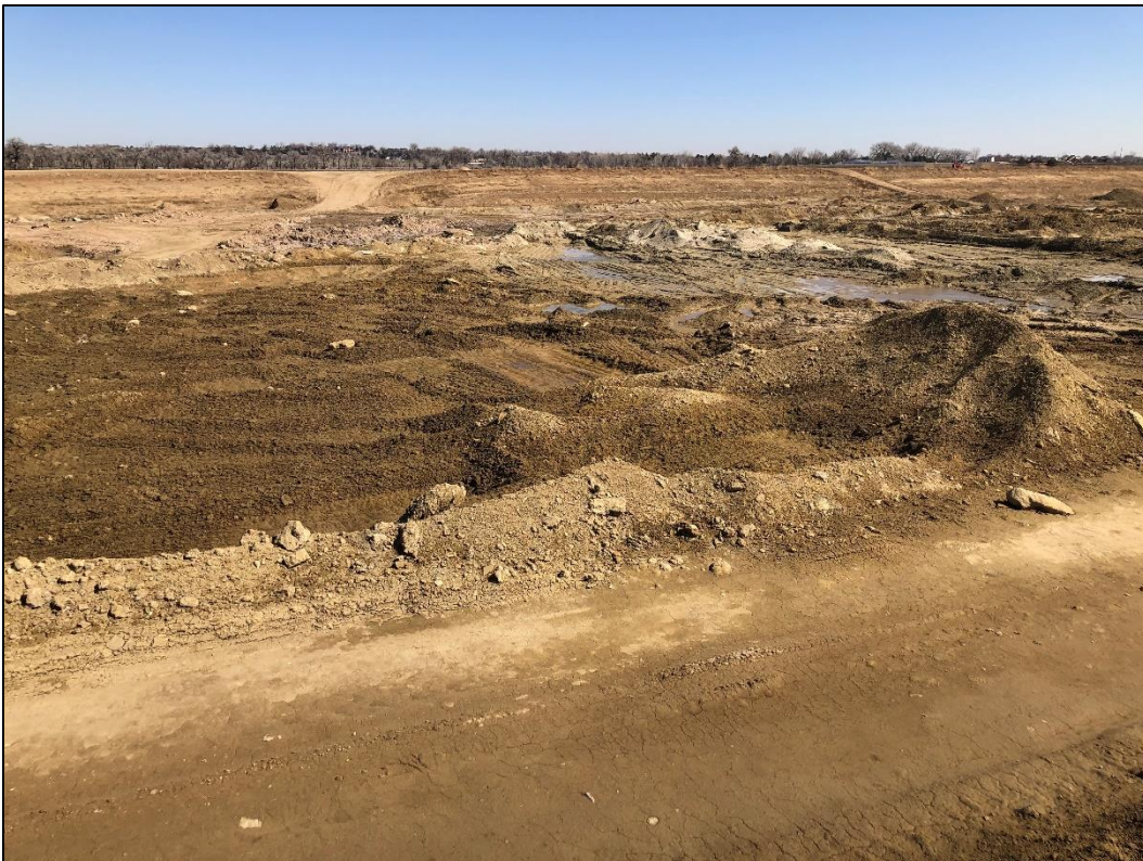
Photo 22. View looking north across central portion of new (unauthorized) reservoir pit. Note various material stockpiles on pit floor and some standing water.
