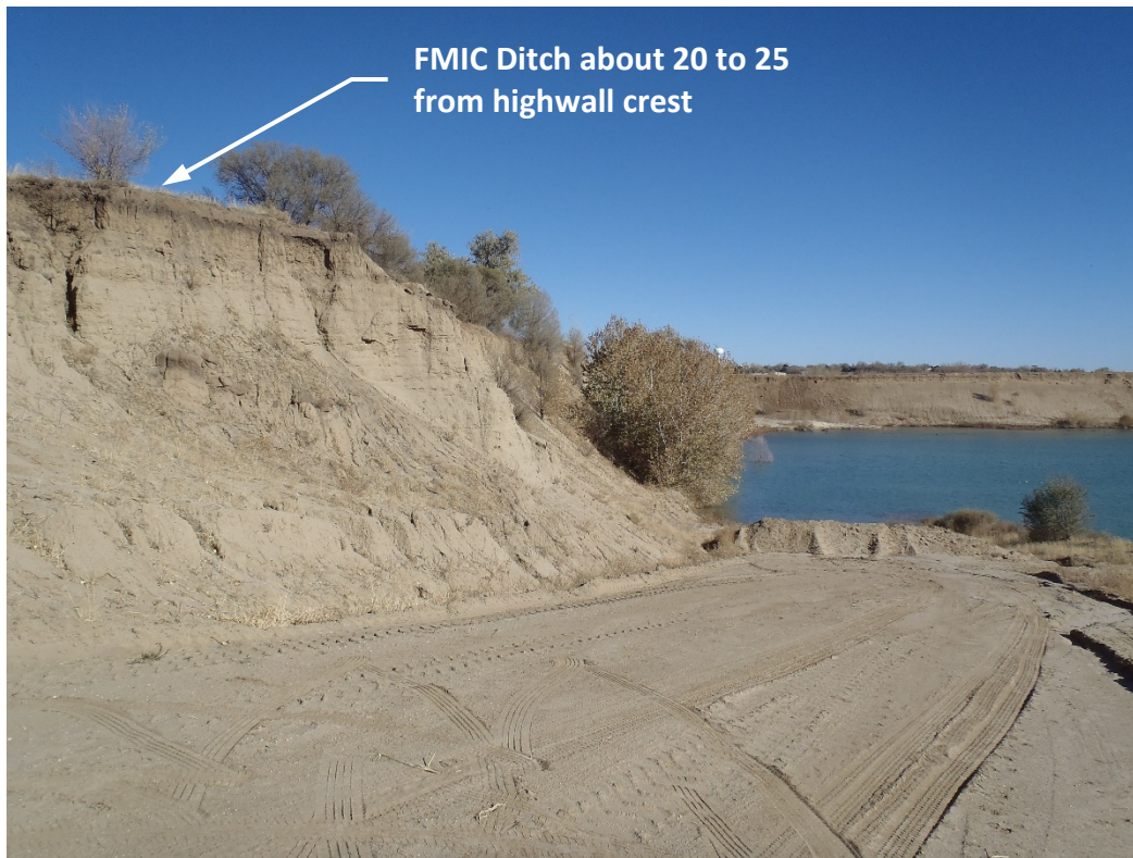
Photo 3. Highwall slope steeper than 1H:1V (looking east from NW corner of new wash pond).
