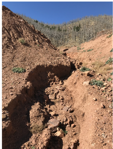
3. GULLY DIVERTS RUNOFF TO SLIDE AREA
