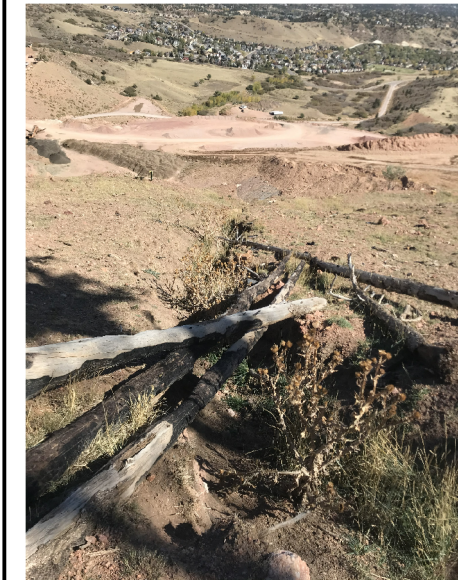
6. GULLY DIVERTS RUNOFF TO SLIDE
