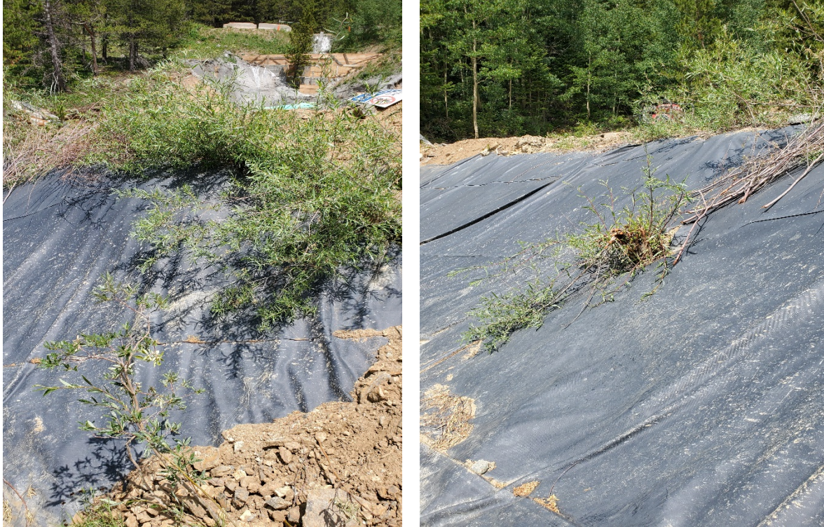
Bushes penetrating liner causing large unrepairable holes.
