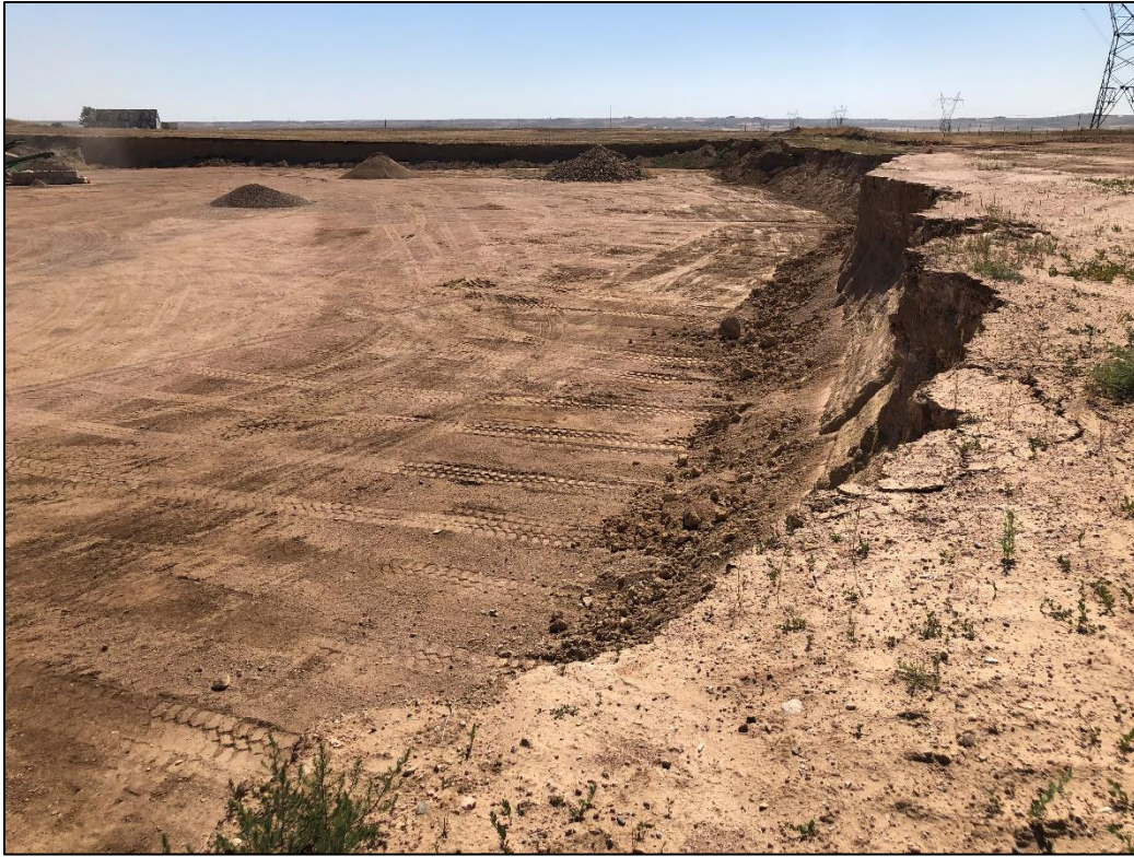
Photo 1. View looking east across southeastern pit wall approximately 15-18 feet in height with near vertical slopes.
