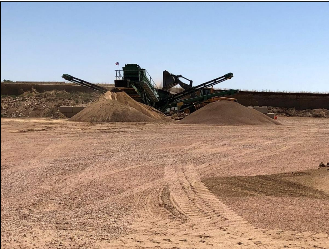
Photo 4. View looking east across central portion of pit, showing portable processing plant active on pit floor during inspection.
