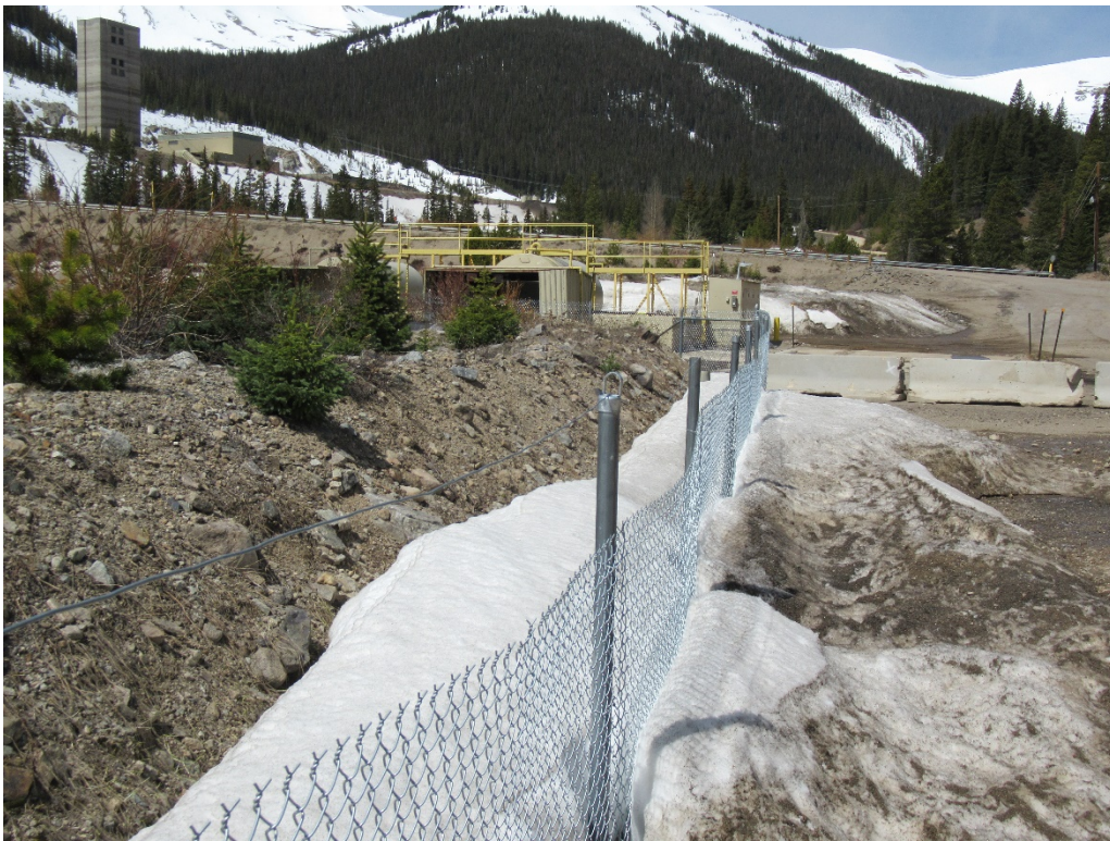
View of damaged fence around EPF 1.2
