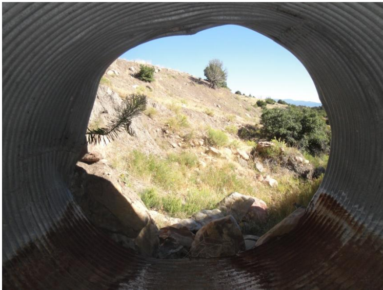
Picture 2. Damaged outlet of 8.8 ft. culvert.
