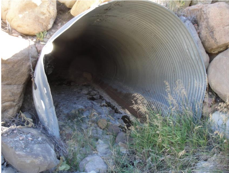
Picture 1. Damaged inlet of 8.8 ft. culvert.
