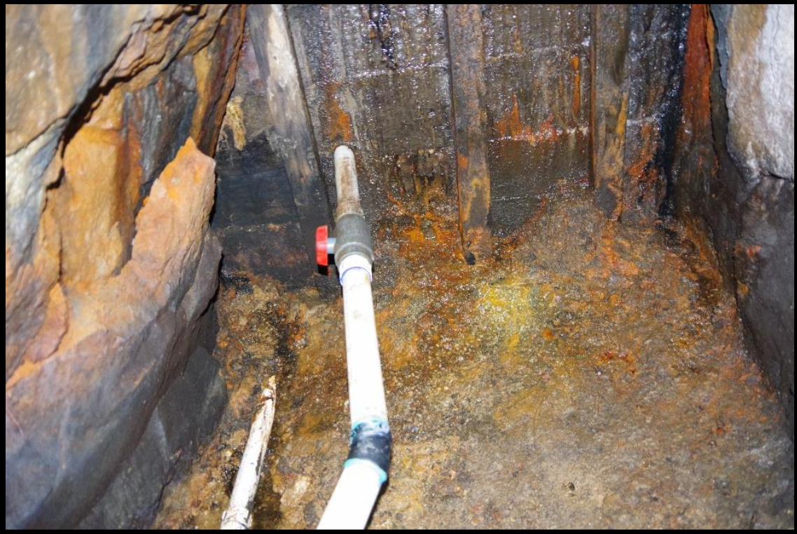
Photo 10: Lower piping in bulkhead; Note closed valve and precipitant on floor
