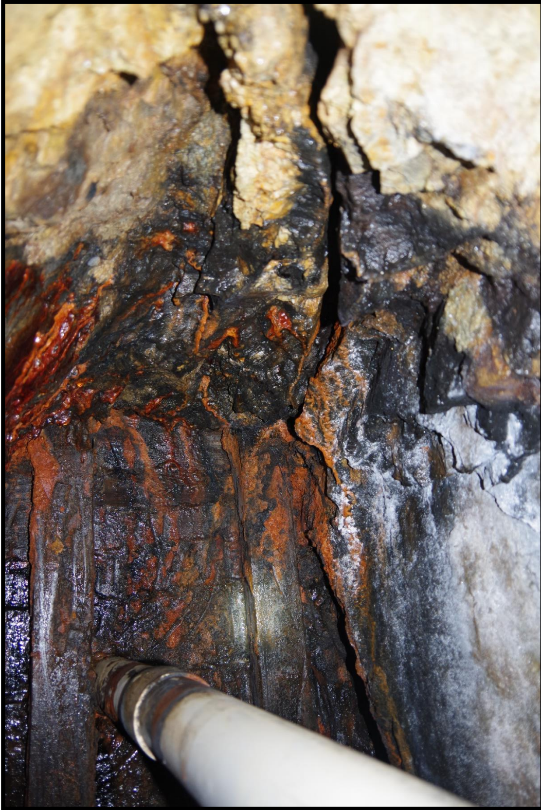
Photo 12: Upper bulkhead piping and extent of dripping along vein in back
