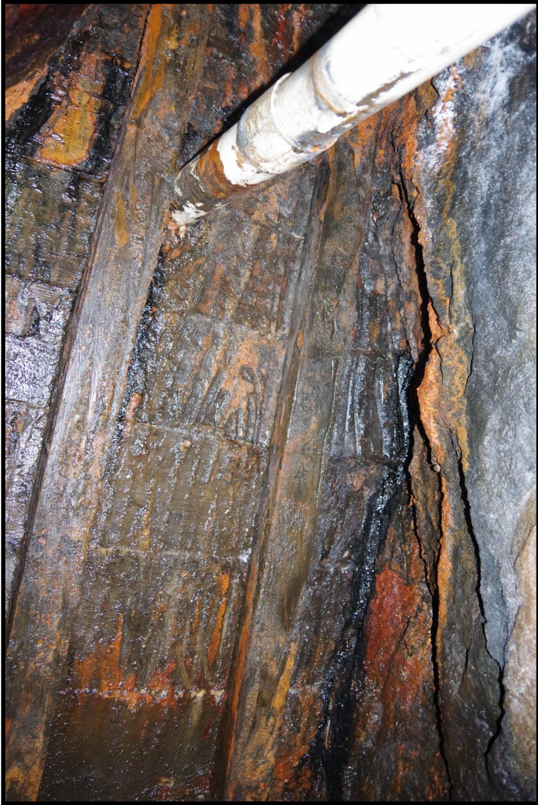
Photo 13: Seepage along right side of bulkhead
