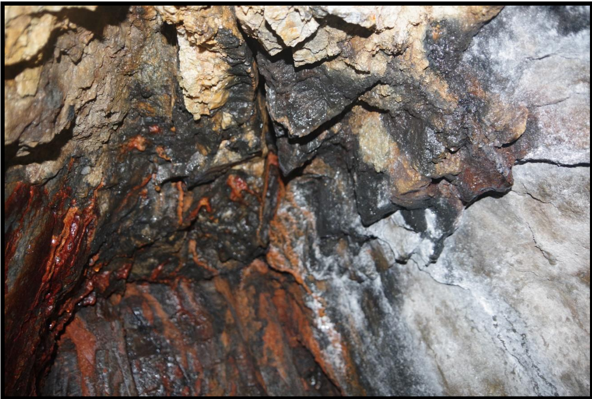
Photo 11: Seepage and precipitant at top of bulkhead
