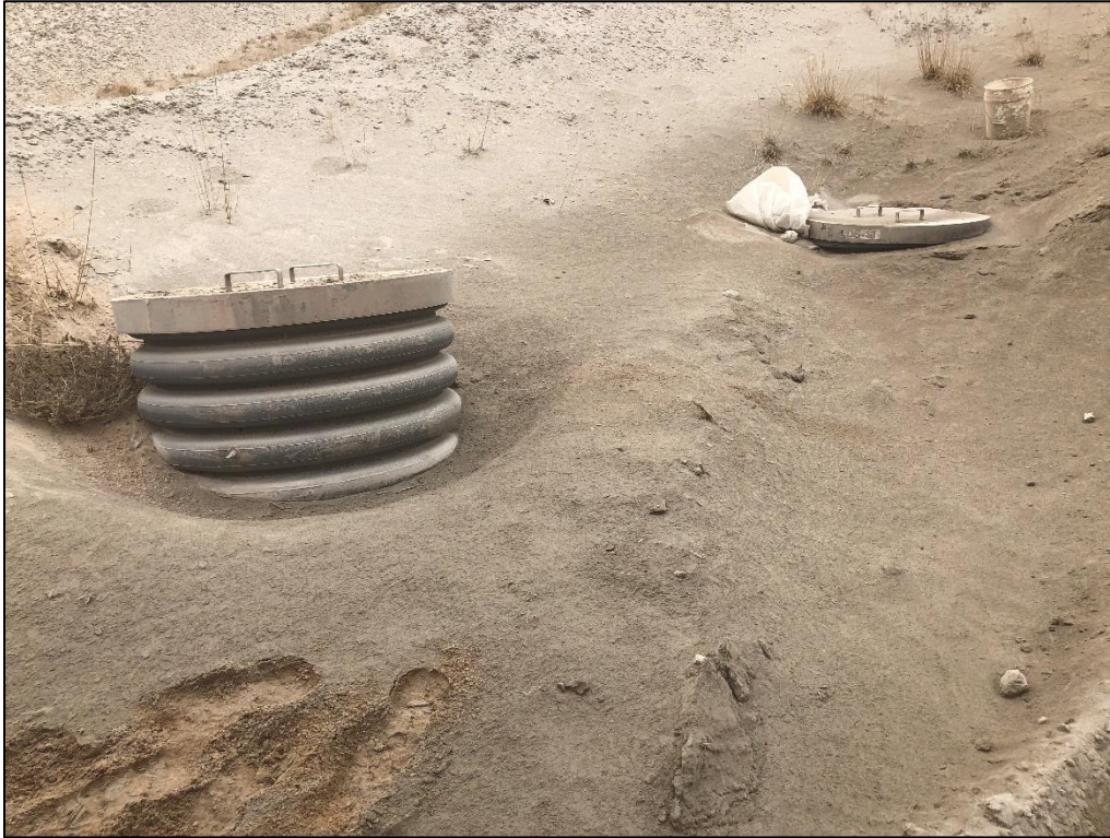
Photo 15. View looking north, showing location of LDS sumps AG-LDS-12 (foreground) and AG-LDS-13 (background) at northern edge of crusher area in Phase IV of AGVLF.
