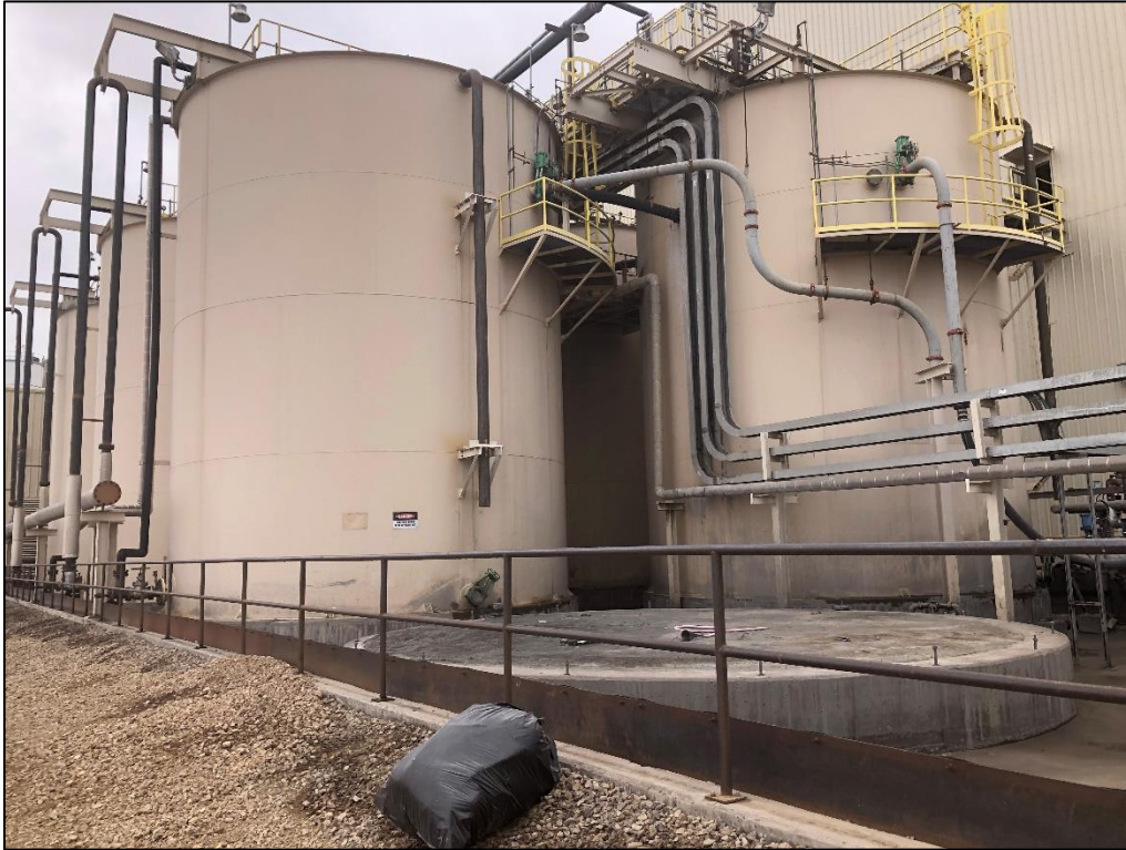
Photo 27. View looking across vat leach circuit present on west side of HGM, still offline since February 2018.
