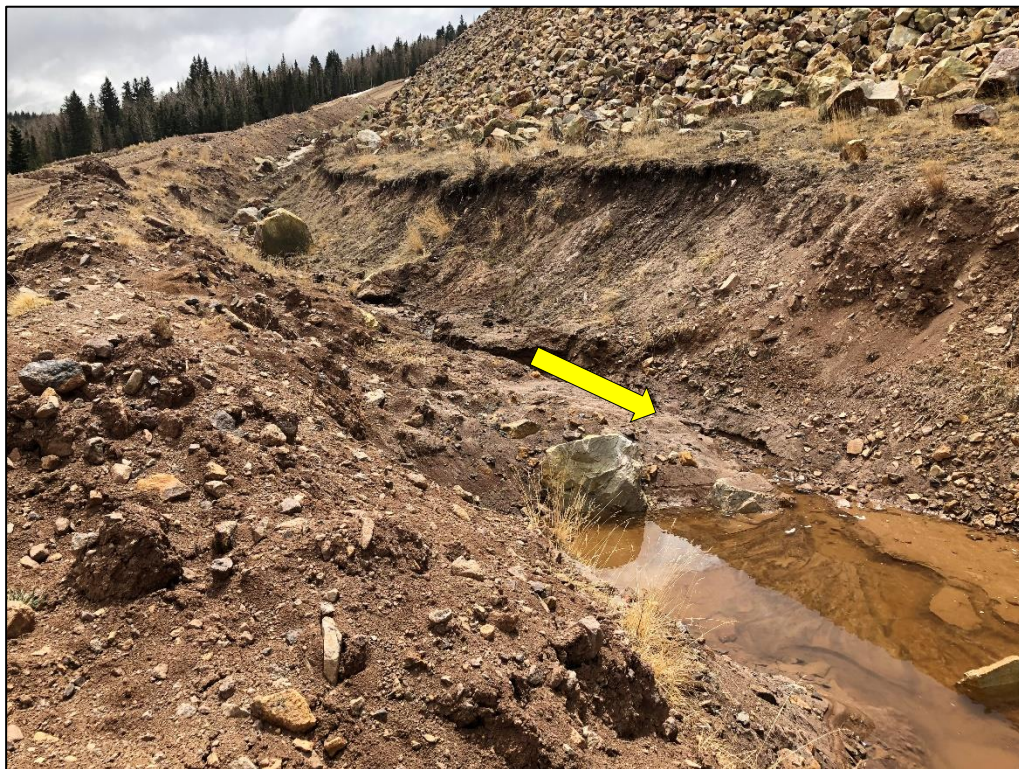
Photo 30. View looking southeast from seep accumulation trench at eastern toe of ECOSA. A trickle of water was flowing into the trench during the inspection (flow direction indicated).
