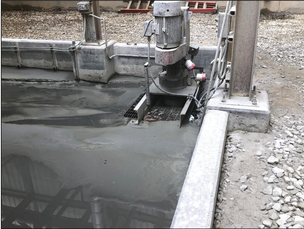
Photo 23. View looking across secondary containment for processed ore thickener, located on east side of HGM. High pH thickener discharge was draining into sump (shown) located at northwest corner of this structure.
