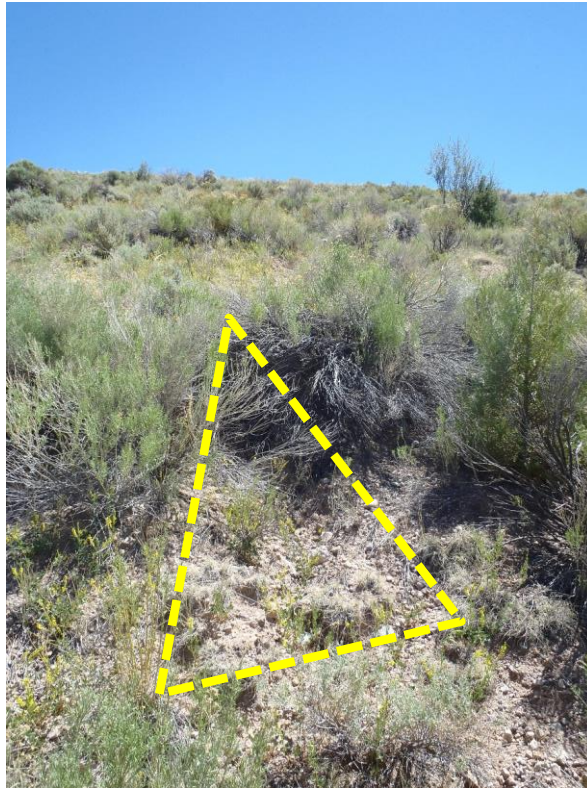
Photo 3. Typical erosion gully observed on the north end of the downstream slope (looking upslope).
