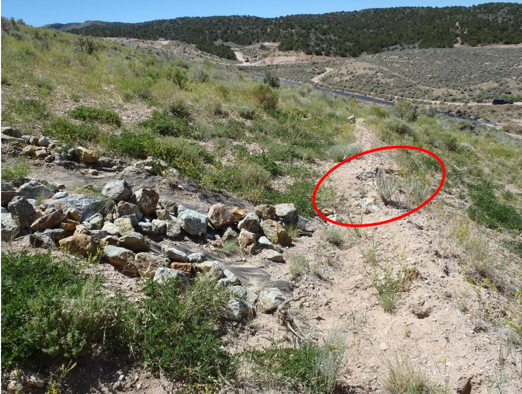
Photo 7. Drainage repair (cross channel) needing maintenance (some cross channels eroded right banks).
