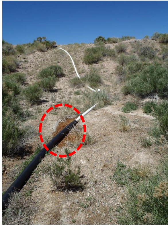
Photo 9. Leaking pump back line (north end of beach, looking west).
