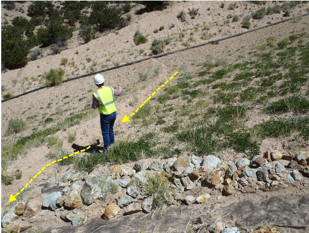
Photo 5. Drainage repair (cross channel) needing maintenance (some cross channels eroded right banks).
