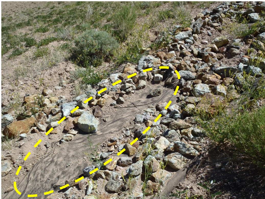
Photo 4. Drainage repair work (downchute) needing maintenance (note exposed geotextile filter).
