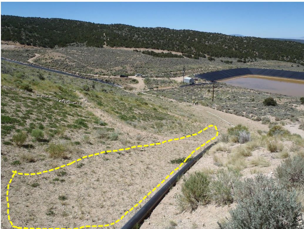
Photo 8. Vegetation not fully established, north end of previously completed erosion repairs (looking SW).
