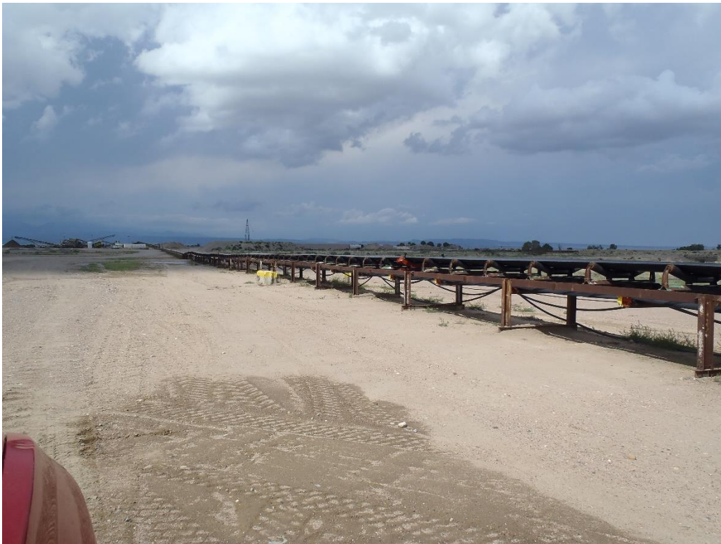
Photo 4. Conveyor system, screen plant beyond on left (looking NE).
