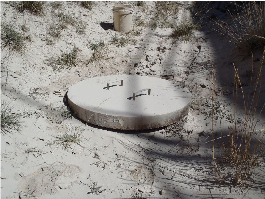
Photo 12. VLF1 LDS13 low profile requires a raise or barrier to prevent debris and meteoric water inflow.
