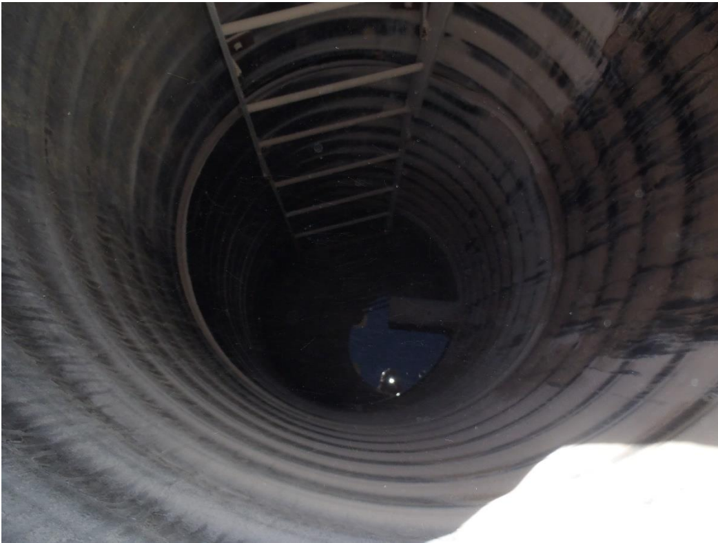
Photo 11. Water observed in VLF1 LDS13 sump.
