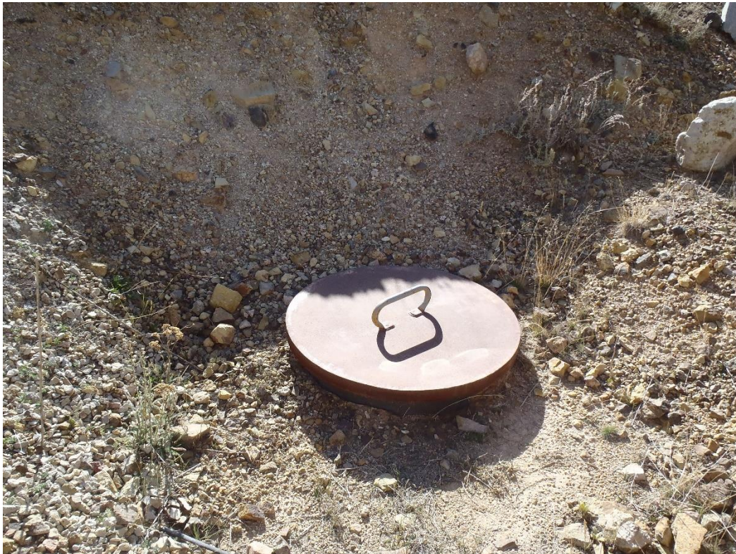
Photo 9. VLF1 LDS1 low profile requires a raise or barrier to prevent debris and meteoric water inflow.
