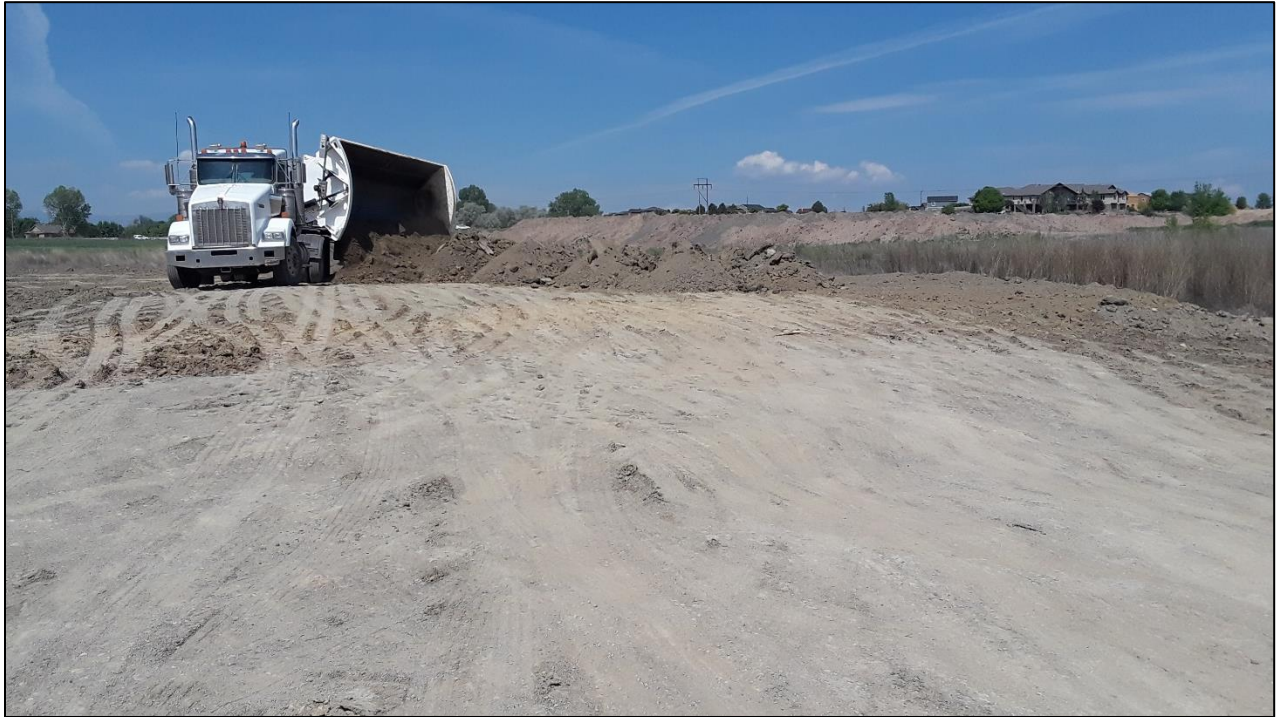
Photo 9. View of truck dumping dirt in the West Reservoir pit during the inspection. TR-4, approved in 2017, allows the operator to backfill pits west of the embankment with inert materials.
