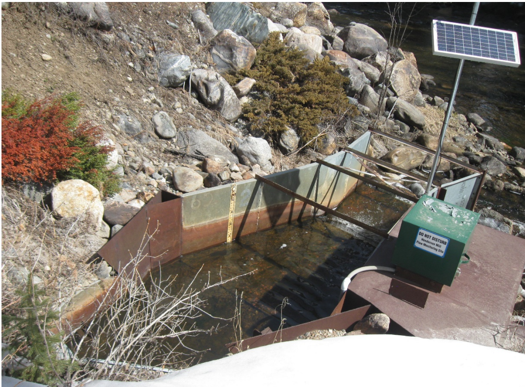
2. East Branch Reservoir - Stormwater diversion discharge point.
