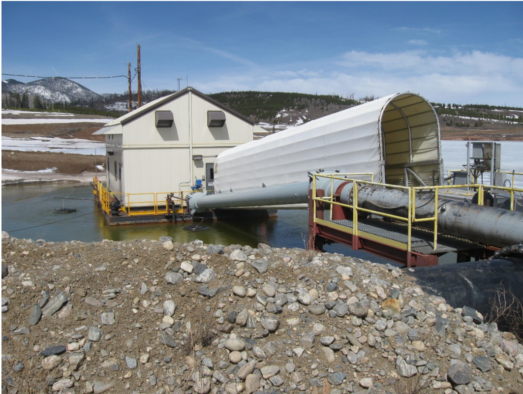
3. Tailings Storage Facility - Barge pump station.
