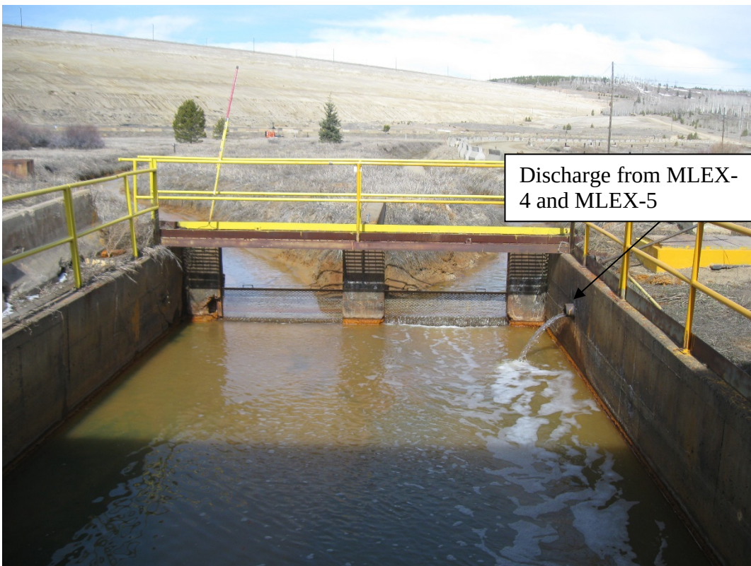
6. Seep Water Collection - Diversion ditches discharging to Ute Park Pump Station.
