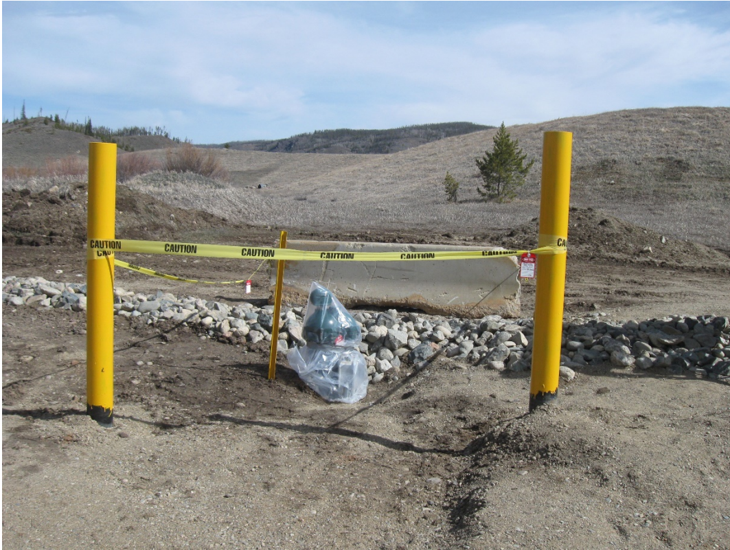
7. Groundwater Intercept System - Pending repair on MLEX-4.
