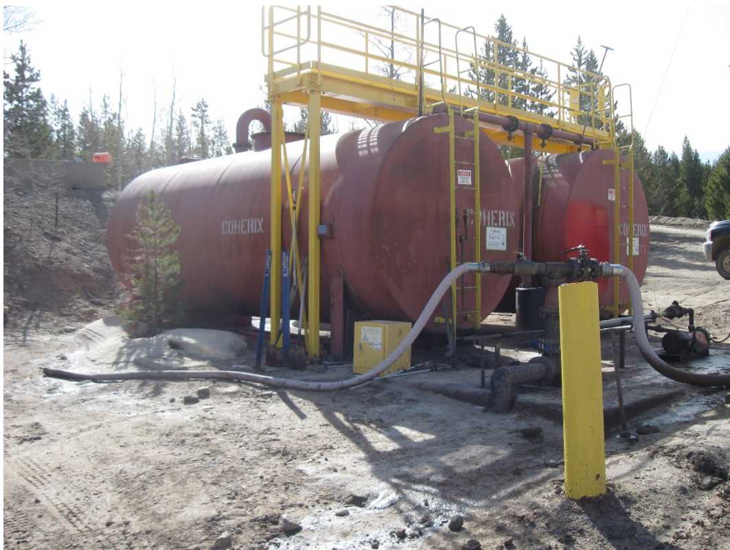
8. Coherex Storage Tanks.
