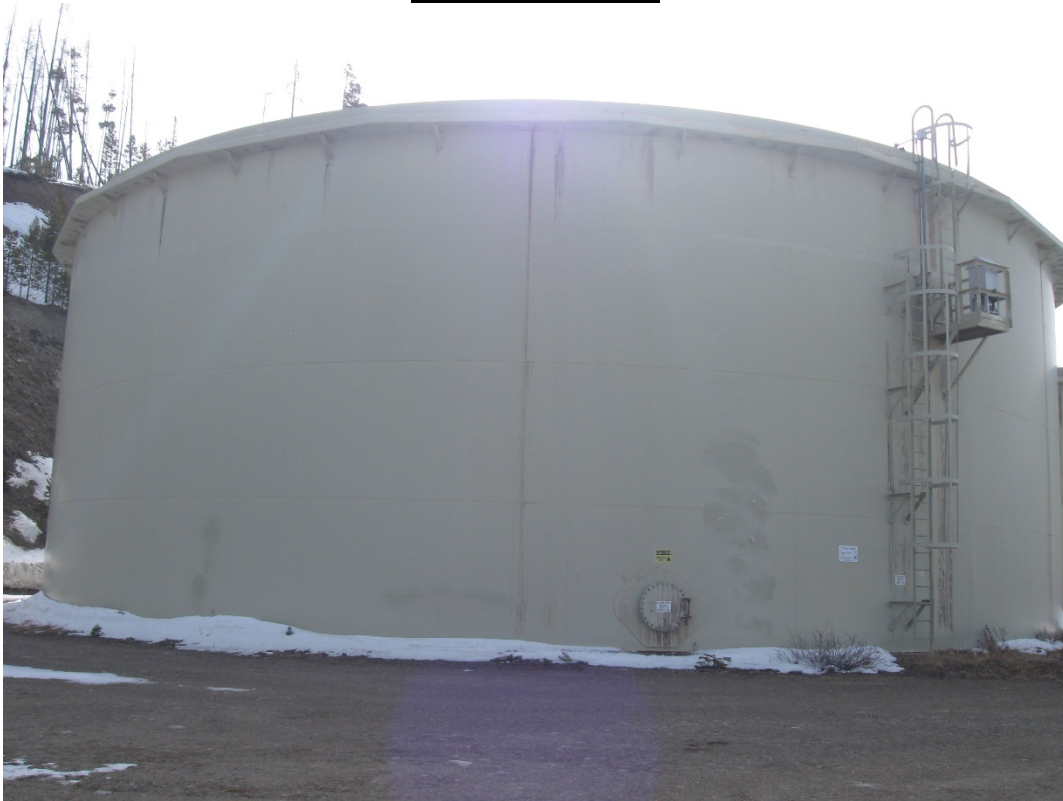
1. Process Water Storage tank.
