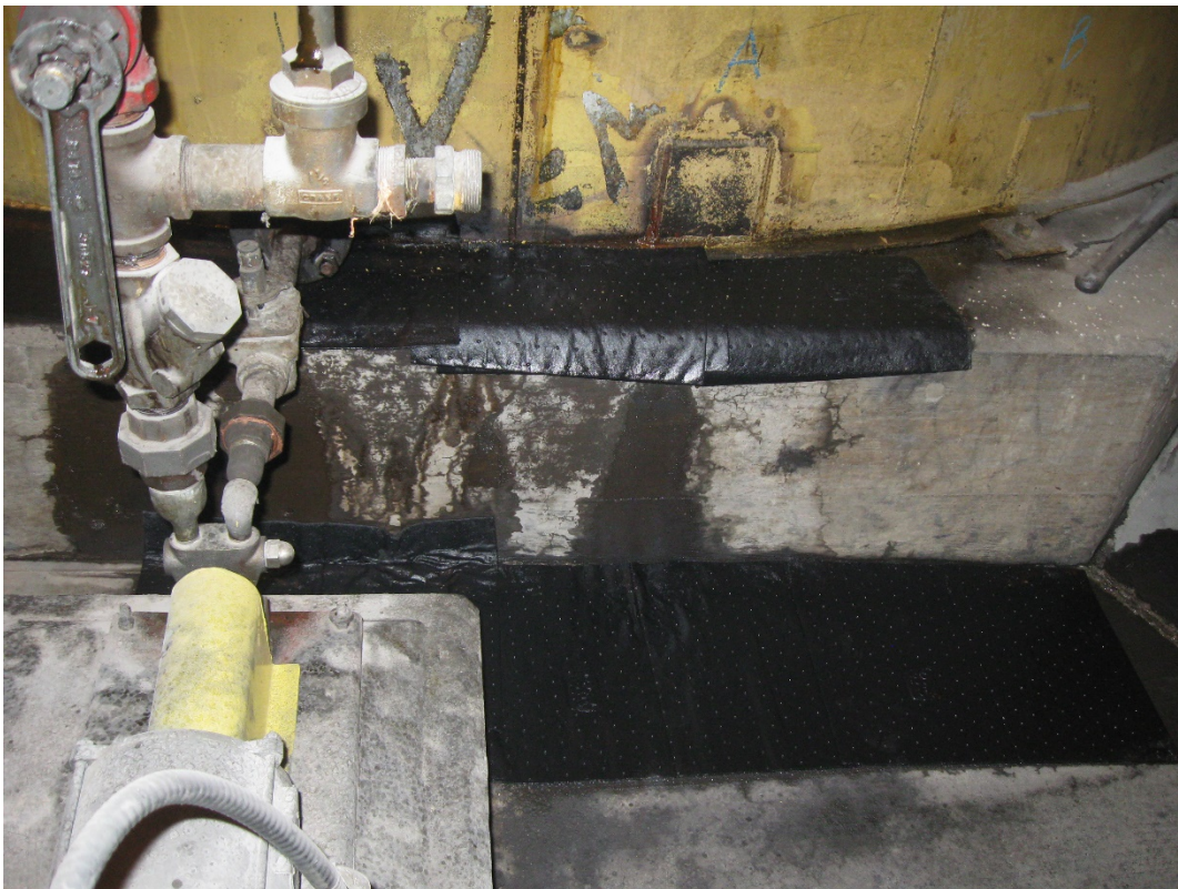
10. Absorbent pads at base of Pine Oil Storage tank.
