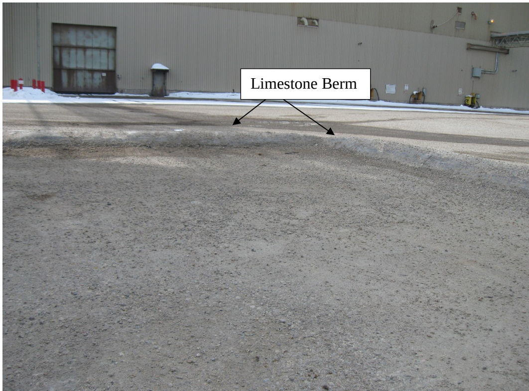
4. Secondary containment for Hydrochloric Acid Storage Area.
