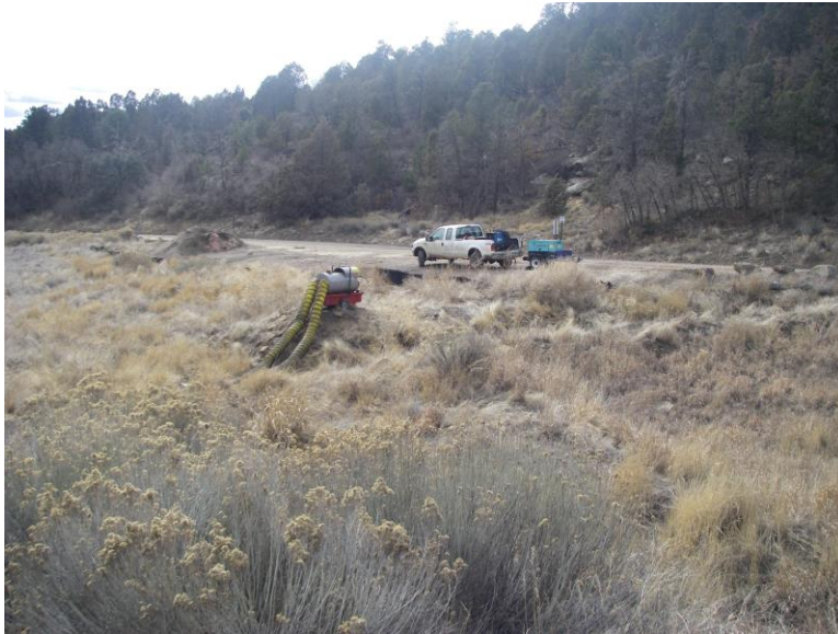
Heating equipment at King II Pond
