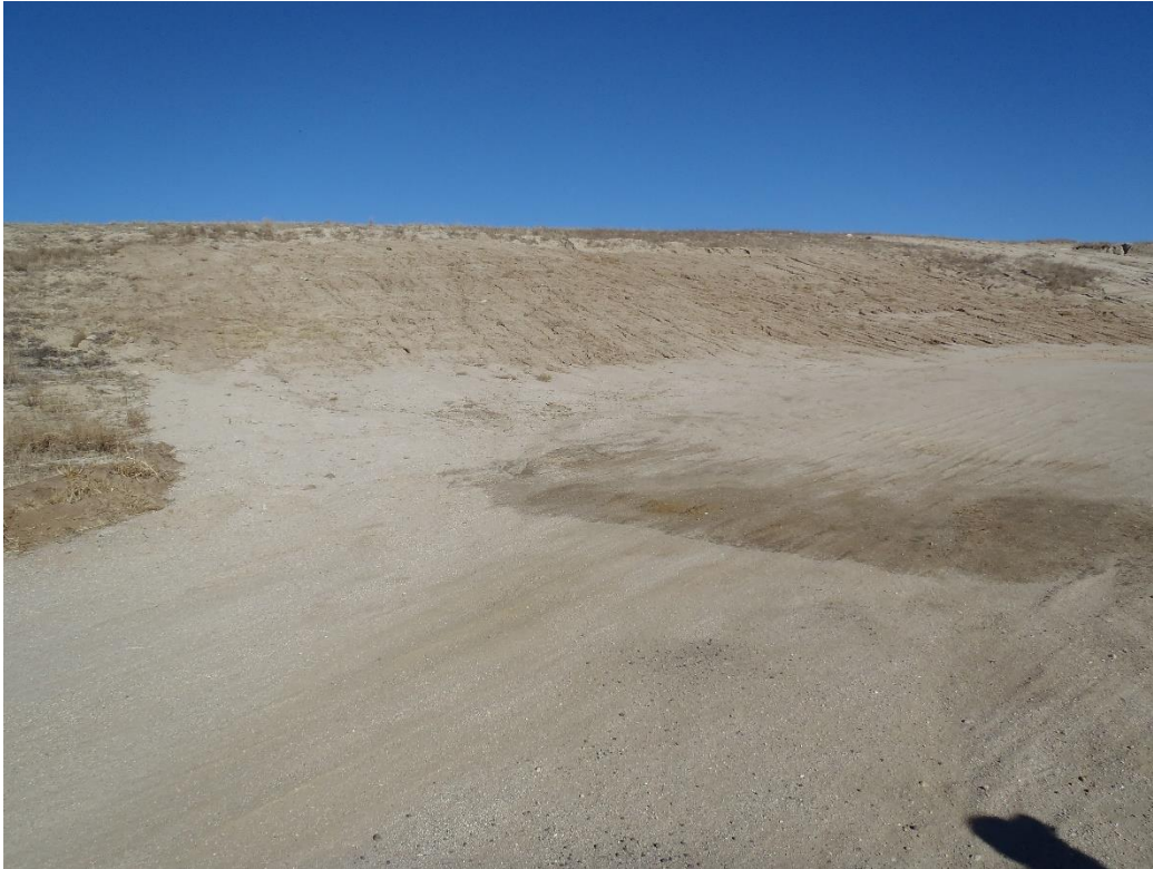
Photo 4. Eroded recently placed topsoil where BMPs are recommended (looking NE).
