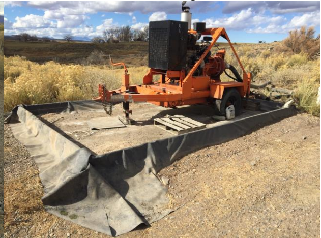
Photo 4 – Pump at Pond NH1 001
