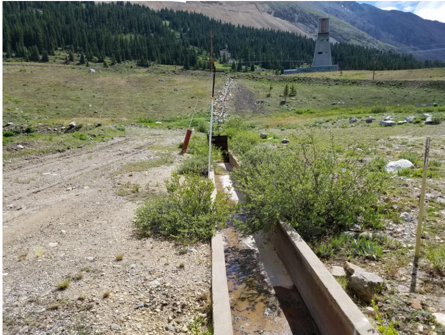
Figure 3. 5-Shaft Pump Station.
