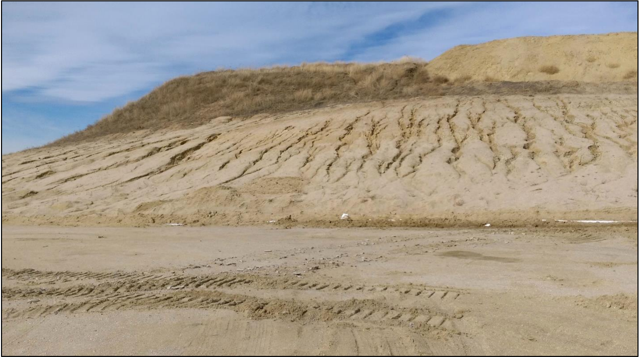
Photo 5. View of western portion of northern pit wall, showing slope gradients of approximately 3H:1V. Note presence of erosional rilling along slope.
