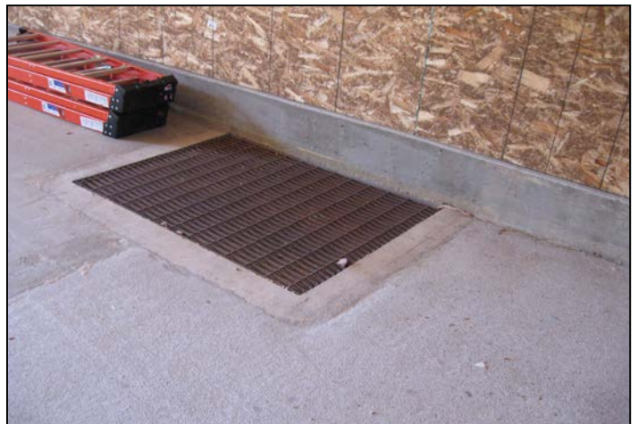
6. Sump in water treatment building.
