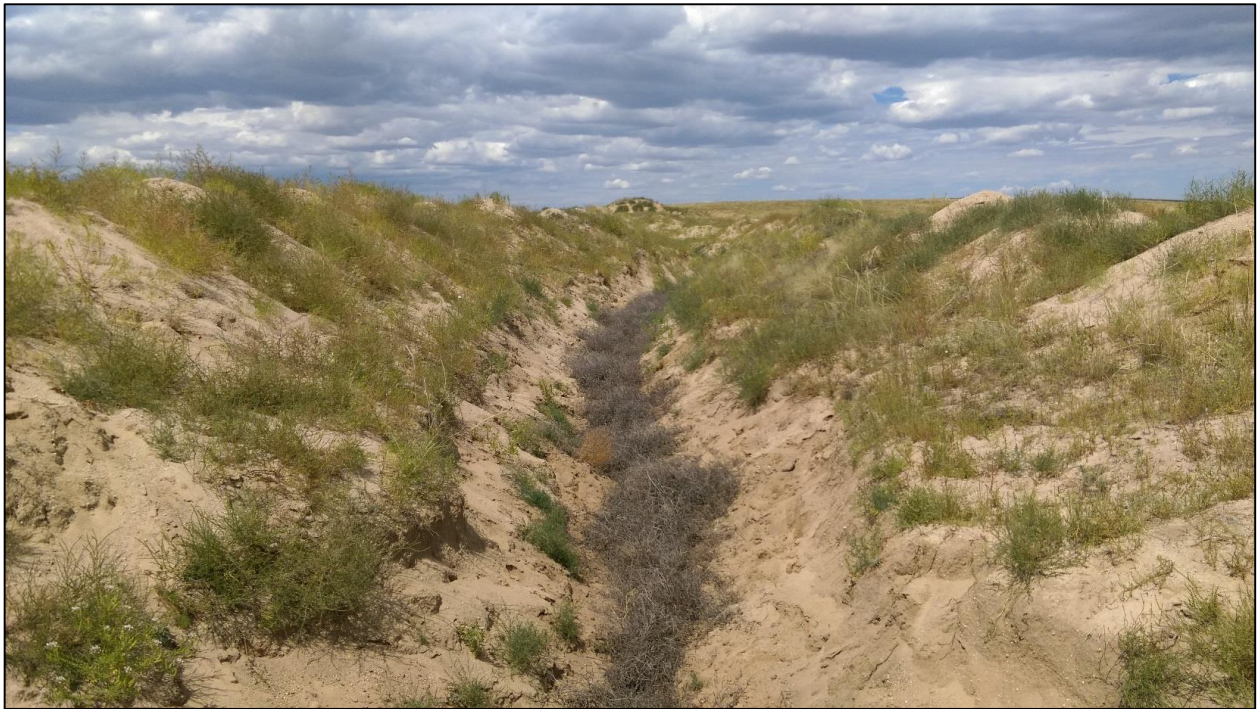
Photo 12. View looking upgradient at portion of drainage downstream of pit, located at southeastern edge of permit area. Note upward slope which does not allow for positive drainage of the pit.
