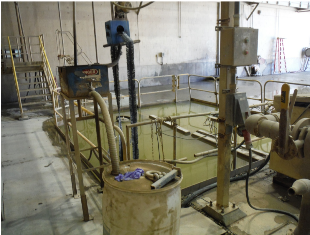
Photo 14. Hydrocarbon skimmer observed at the large vehicle washbay sump in the Ironclad Facility; looking southwest.
