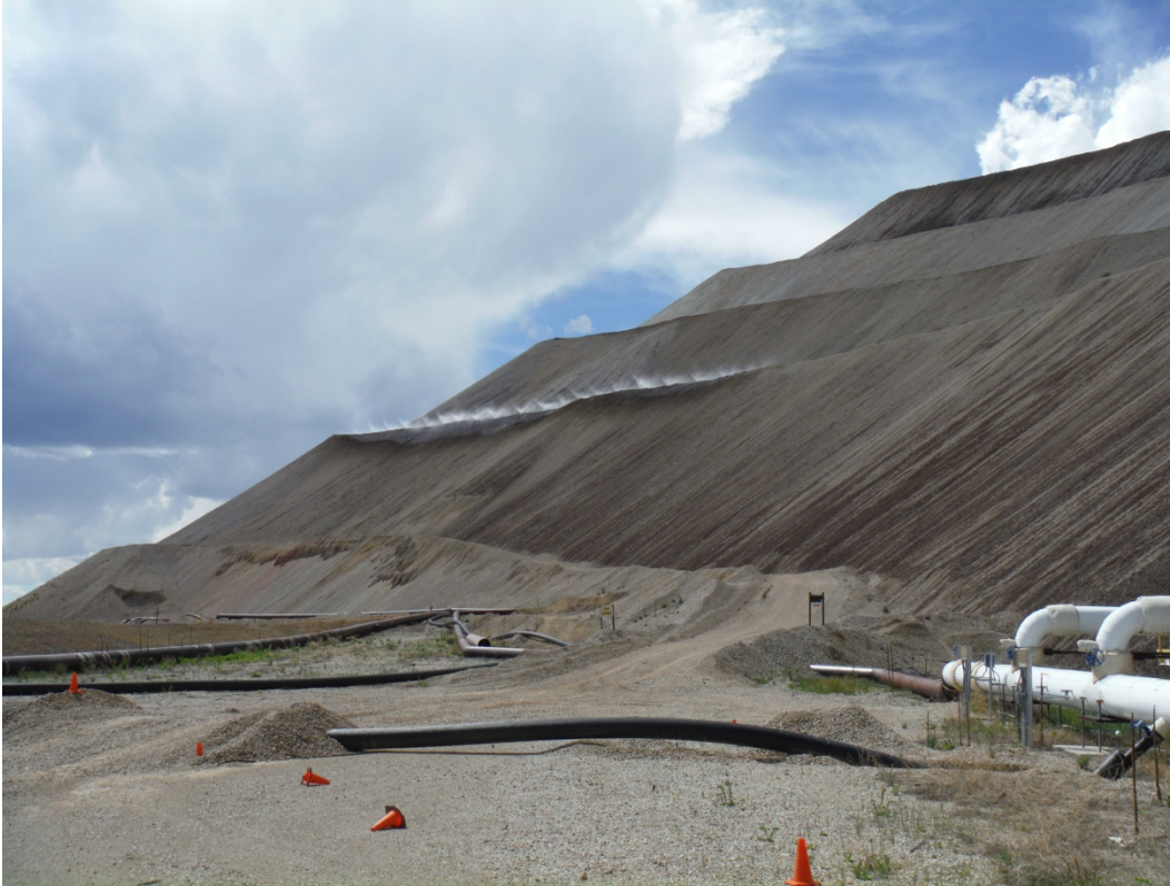
Photo 3. Solution sprinklers on the AGVLF southwest face; looking northwest from the Phase V pumps.
