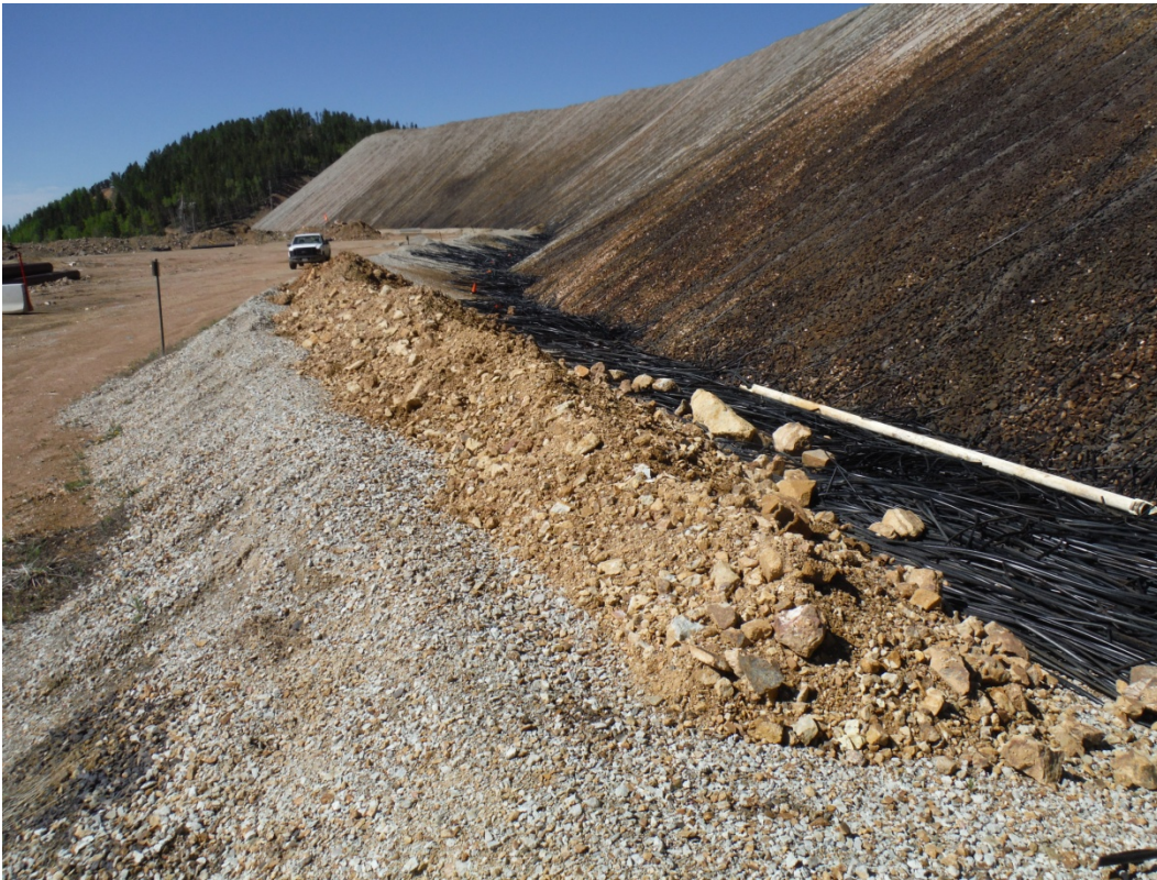
Photo 4. Impacted soil placed over the liner, within the edge of liner berm, from off-liner spill; looking southwest
