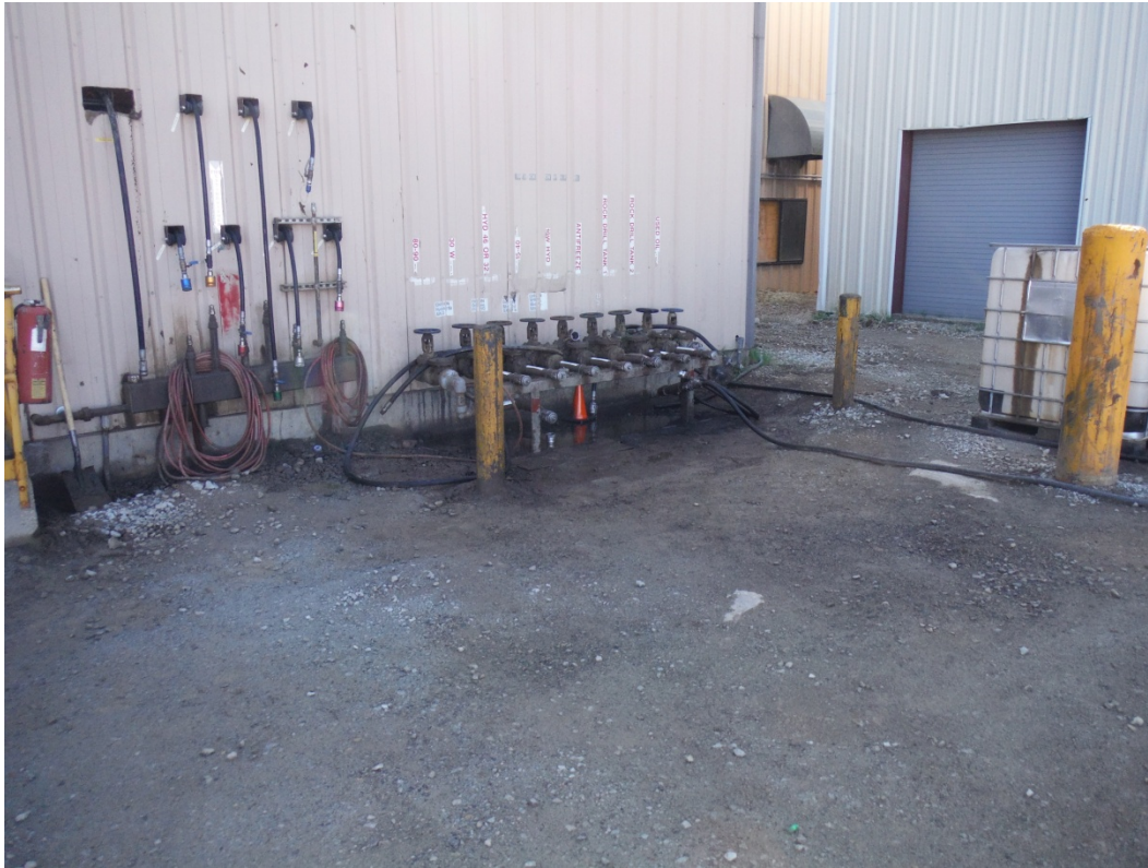
Photo 15. Area of the contaminated soils outside of the Oil Room at the Ironclad Warehouse; looking southeast.
