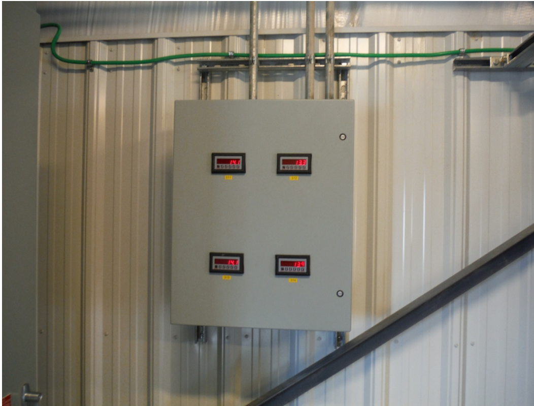
Photo 7. New Phase V PSSA pump gauges; looking northwest.
