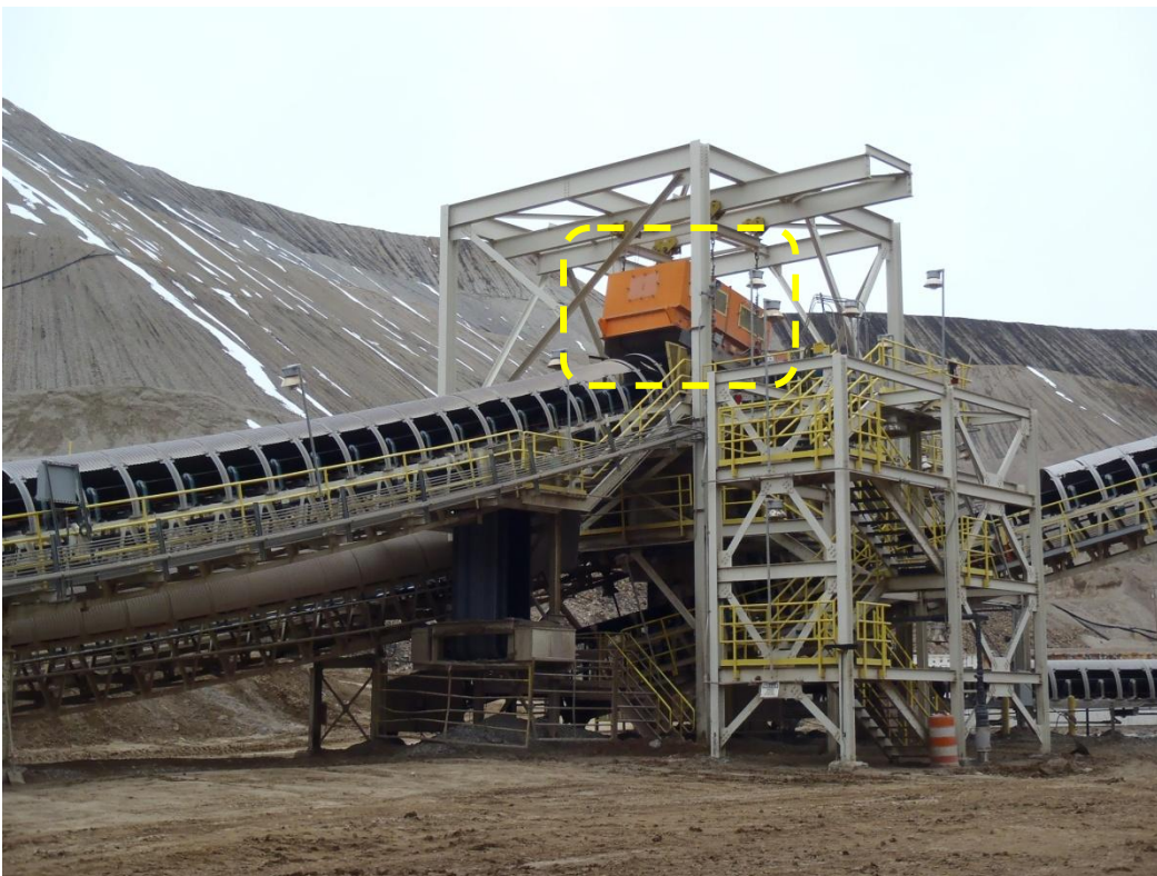
Photo 10. Large electro-magnet used to remove iron and steel from the crushed ore prior to loading the VLF.
