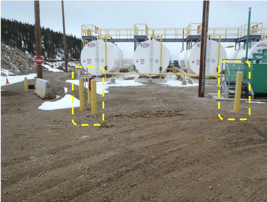
Photo 5. Fuel Island diesel storage tanks over liner with pipe bollards (looking SW).
