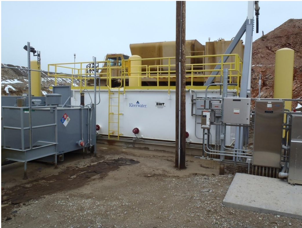
Photo 7. Fuel Island oil/water separator over liner (looking north).
