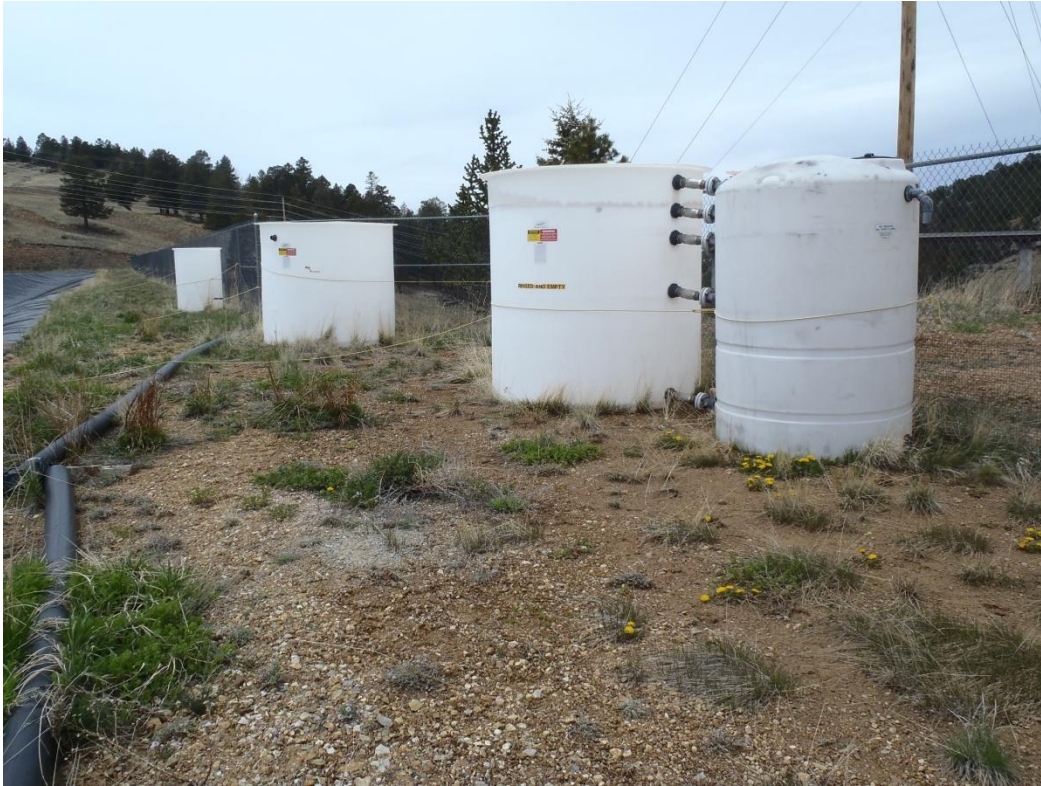
Photo 11. External Storage Pond treatment tanks observed in place on north side of pond.
