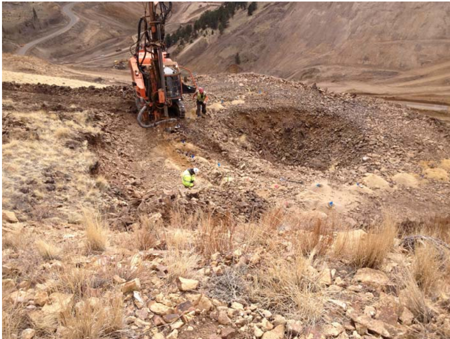
Photo No. 3; Drilling UG #6120, collapsed adit.
