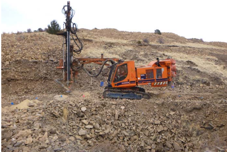
Photo No. 1; Drilling UG #6120, collapsed adit.
