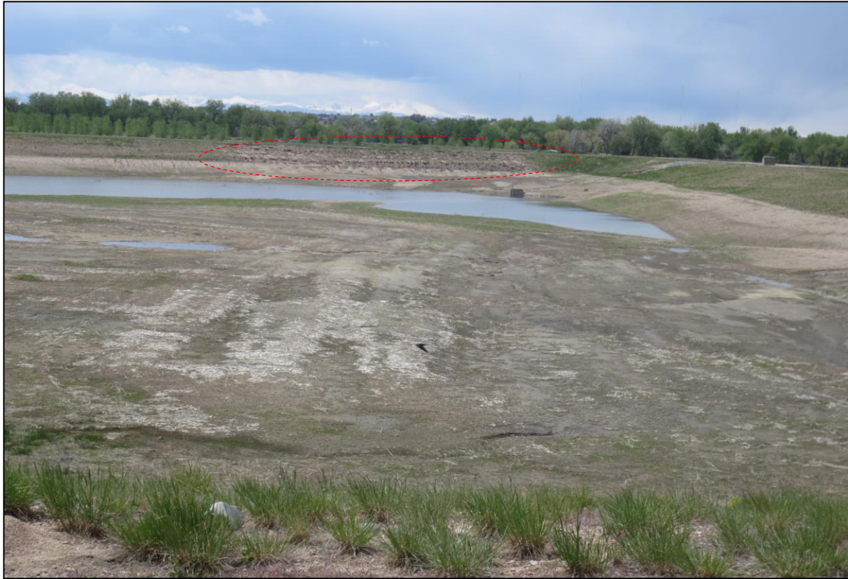
Photo 1: View looking west. Damaged section of the liner in reservoirs A circled in red.
