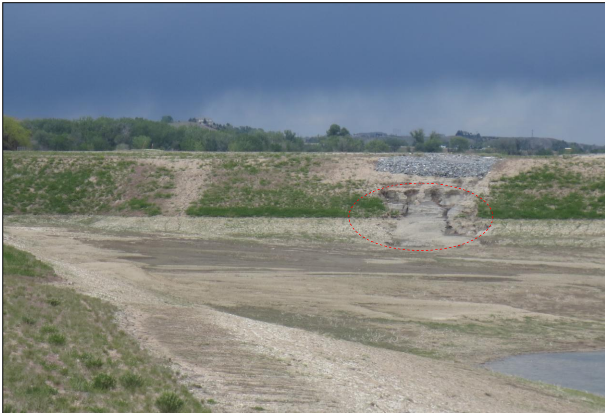
Photo 2: View looking north. Damaged section of the liner in reservoirs A, underneath the emergency spillway circled in red.
