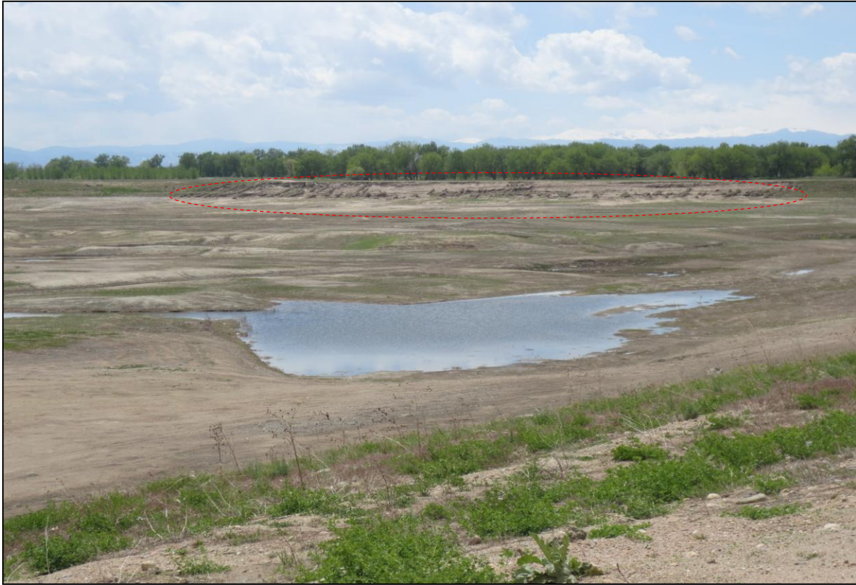
Photo 3: View looking west. Damaged section of the liner in reservoirs B circled in red.
