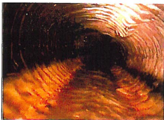
Figure 5 Functioning Solution Collection Pipe w/ 20% Ring Deflection (Binocular Shape)
