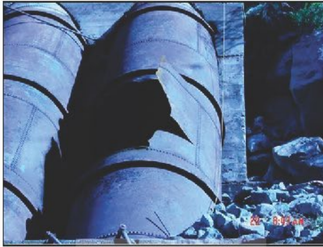
PENSTOCK RUPTURE DAMAGE
