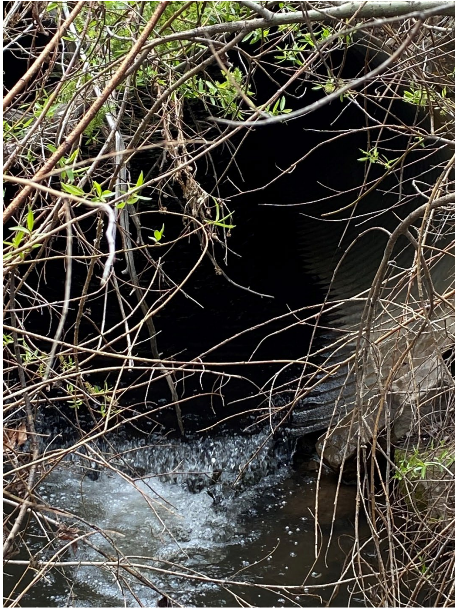
Picture 4: Culvert on Road M44 that is elevated about 1-2 inches above Goat Creek.
