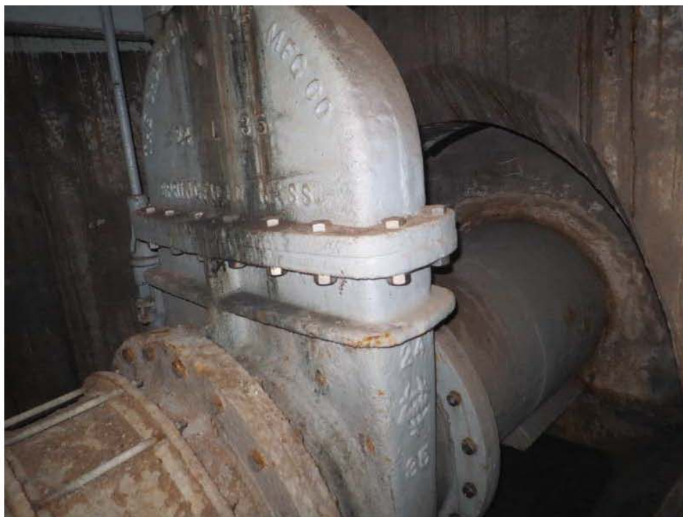
Photo 11 - Outlet works pipe; note bolt corrosion and coating chipping off; 9/9/2021.
