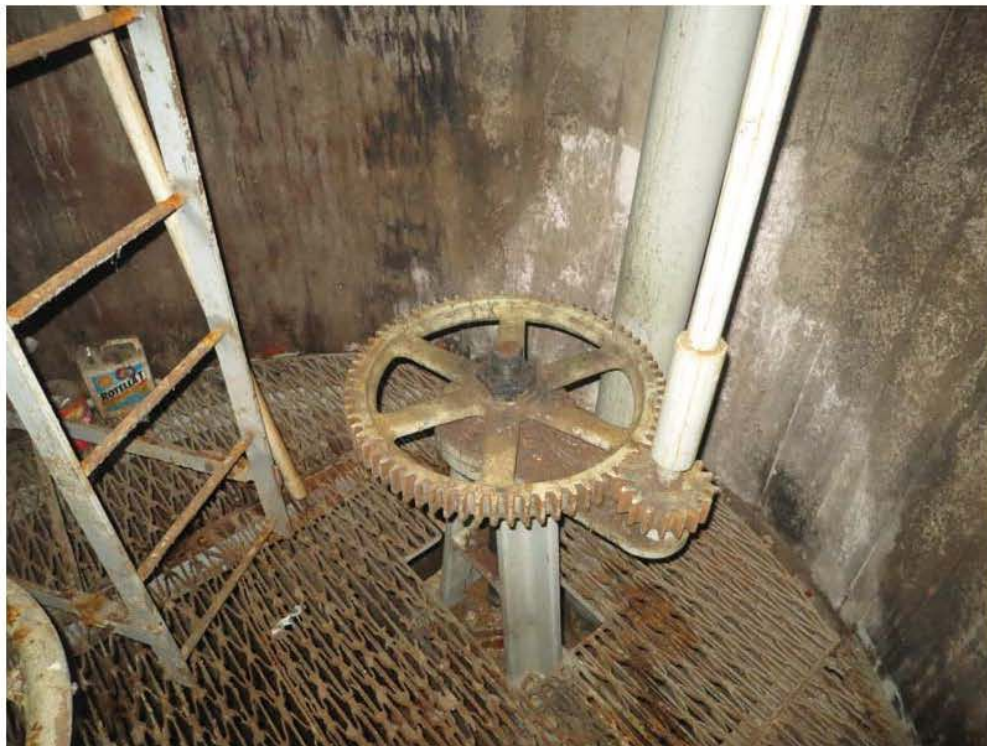
Photo 10 - Regulating gate sprocket in gate chamber; note the metal floor grates are corroded and need to be replaced; 9/9/2021.
