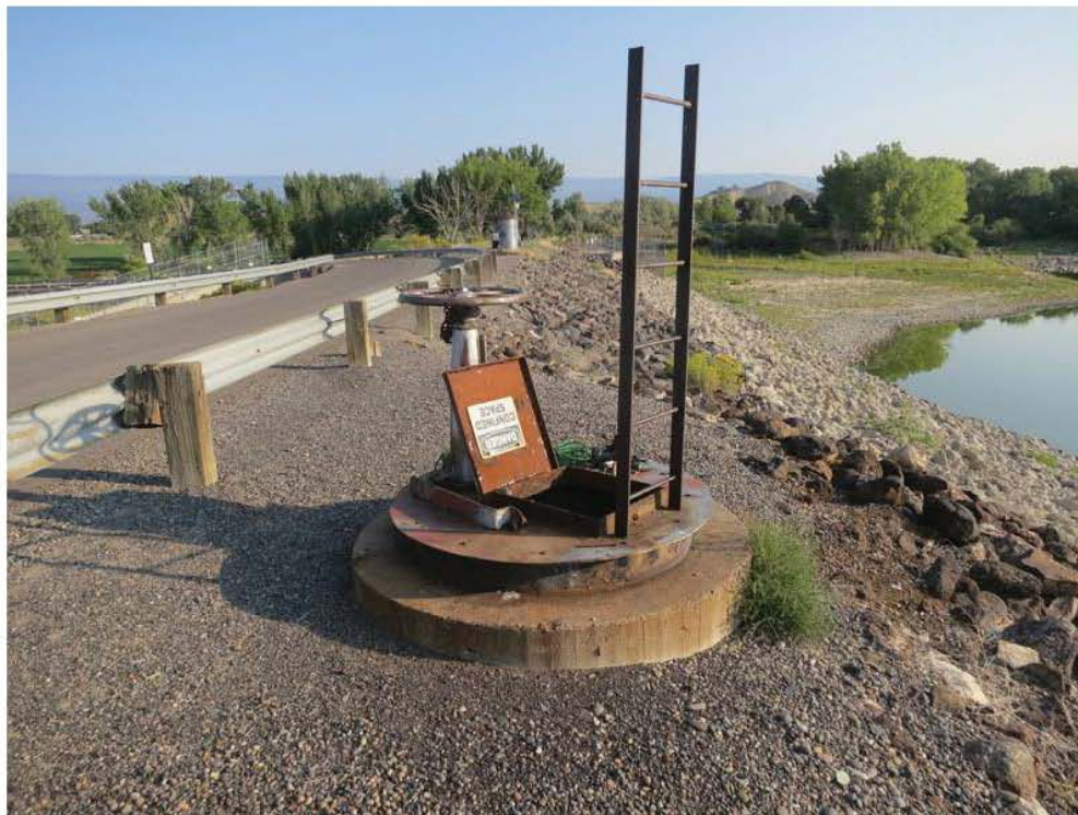
Photo 13 - Gate chamber shaft access; note need to replace gate position indicator on regulating gate operator; 9/9/2021.
