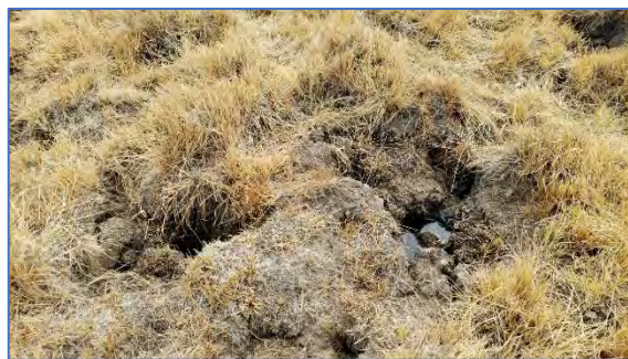
Ditch in need of repair.
