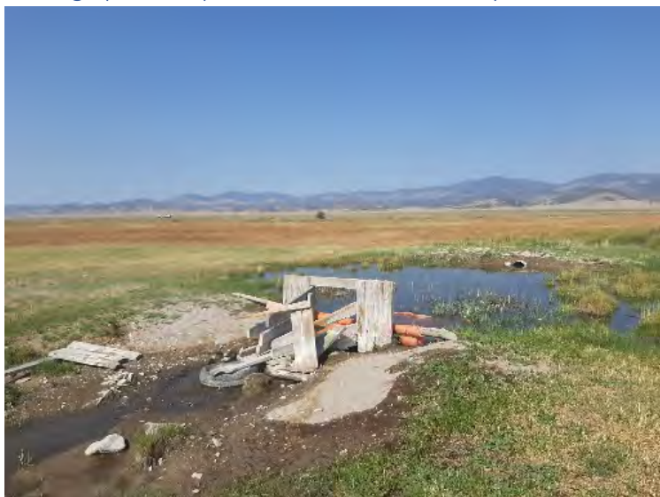
Photograph of dilapidated water control facility.
